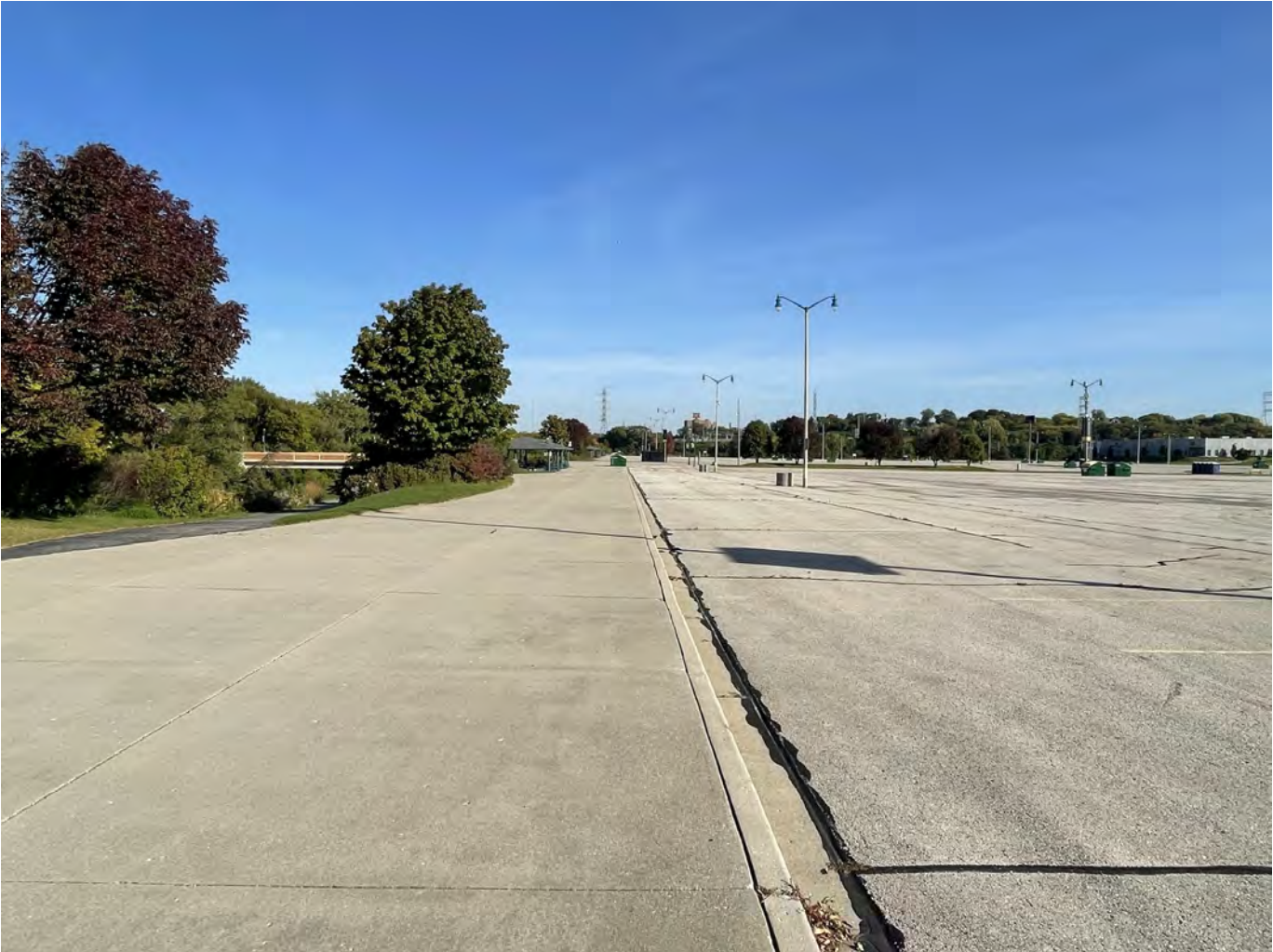
Photo 15: Uecker Lot: Concrete paved plaza and pedestrian path along west side of Uecker Lot (shown on left side of photo): 6-inch concrete pavement overlying 8-inches crushed aggregate. Asphalt paved Uecker Lot (shown on right side of photo): 4-inch asphalt pavement overlying 8-inches crushed aggregate. Photo taken facing north on October 4, 2022.
