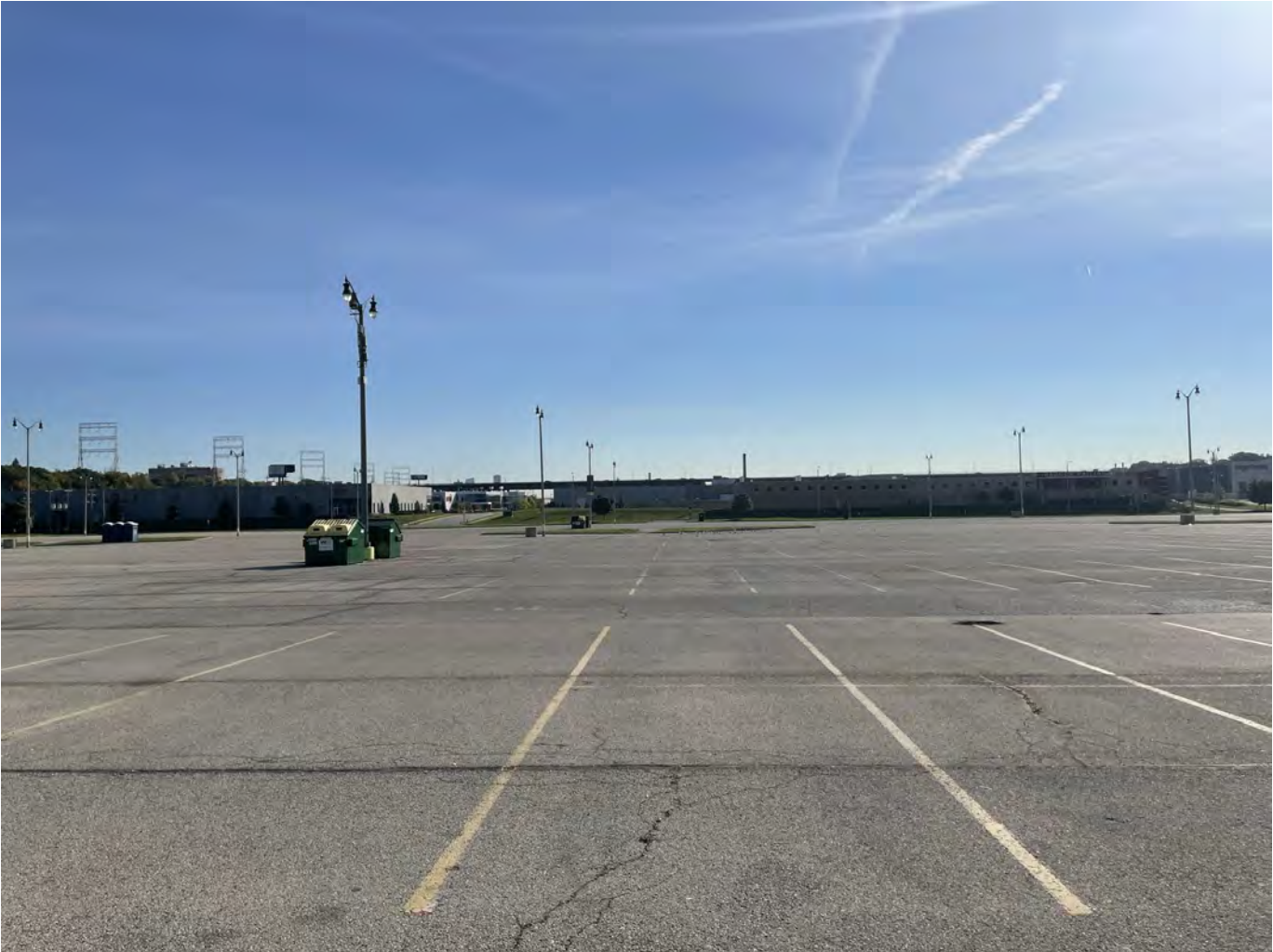
Photo 20: Yount Lot: Asphalt cap over Yount Lot: 4-inch asphalt pavement overlying 8-inches of crushed aggregate base course. Photo taken facing east on October 4, 2022.
