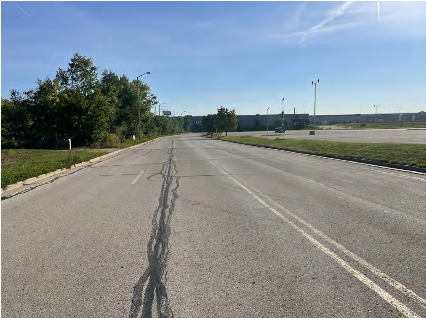
Photo 25: Yount Lot: Asphalt cap over Selig Drive north of Yount Lot: 4-inch asphalt pavement overlying 8-inches of crushed aggregate base course. Photo taken facing east on October 4, 2022.
