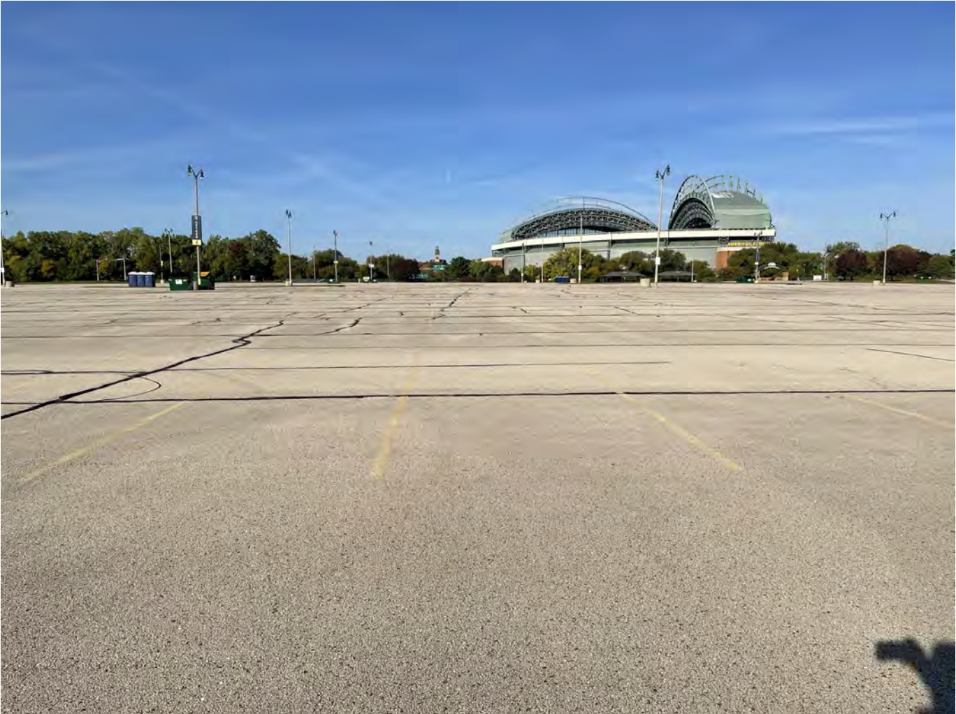
Photo 4: Yount Lot: Asphalt cap over Yount Lot: 4-inch asphalt pavement overlying 8-inches of crushed aggregate base course. Photo taken facing west on October 4, 2022.
