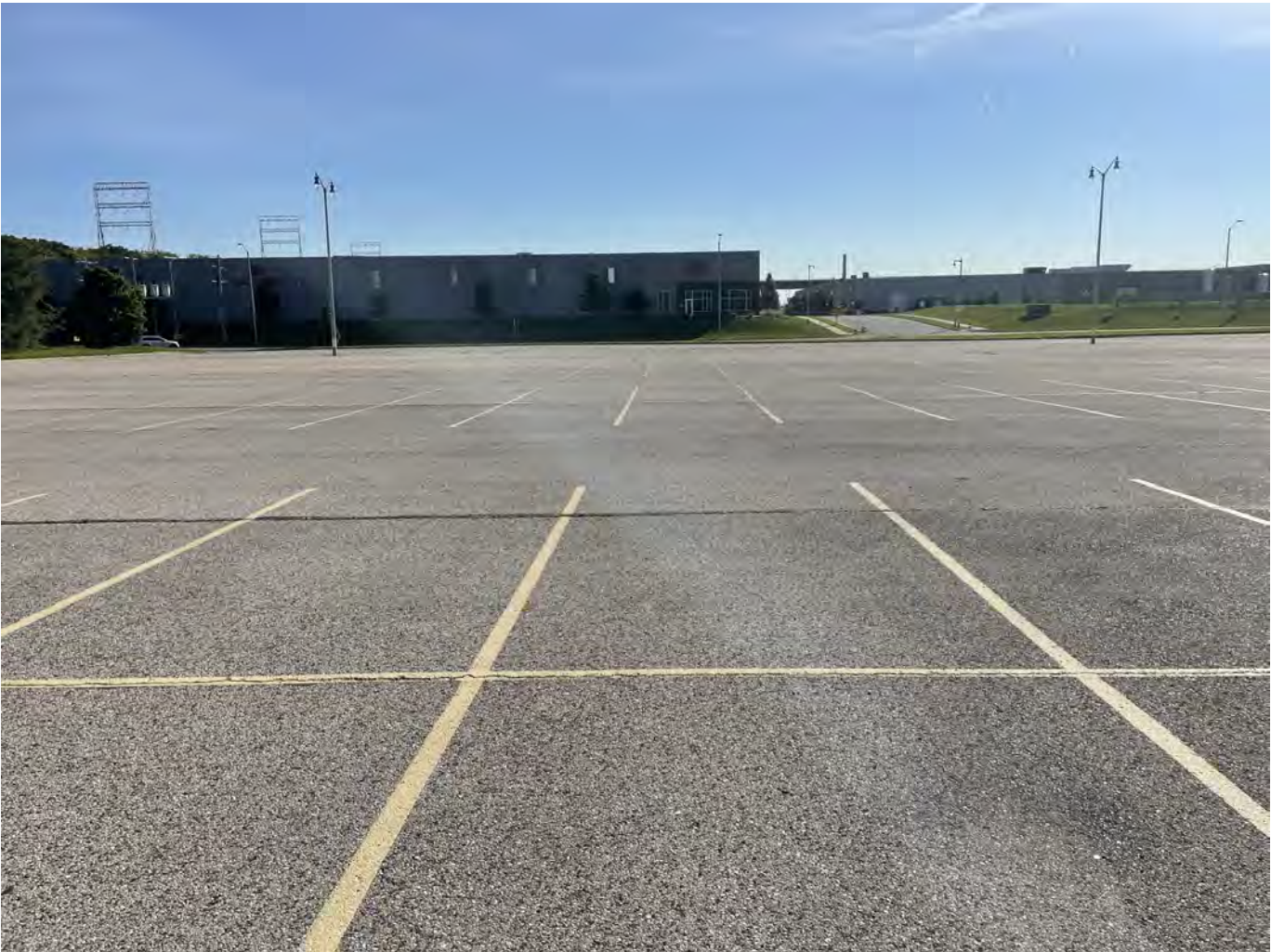
Photo 26: Yount Lot: Asphalt cap over Yount Lot: 4-inch asphalt pavement overlying 8-inches of crushed aggregate base course. Photo taken facing east on October 4, 2022.
