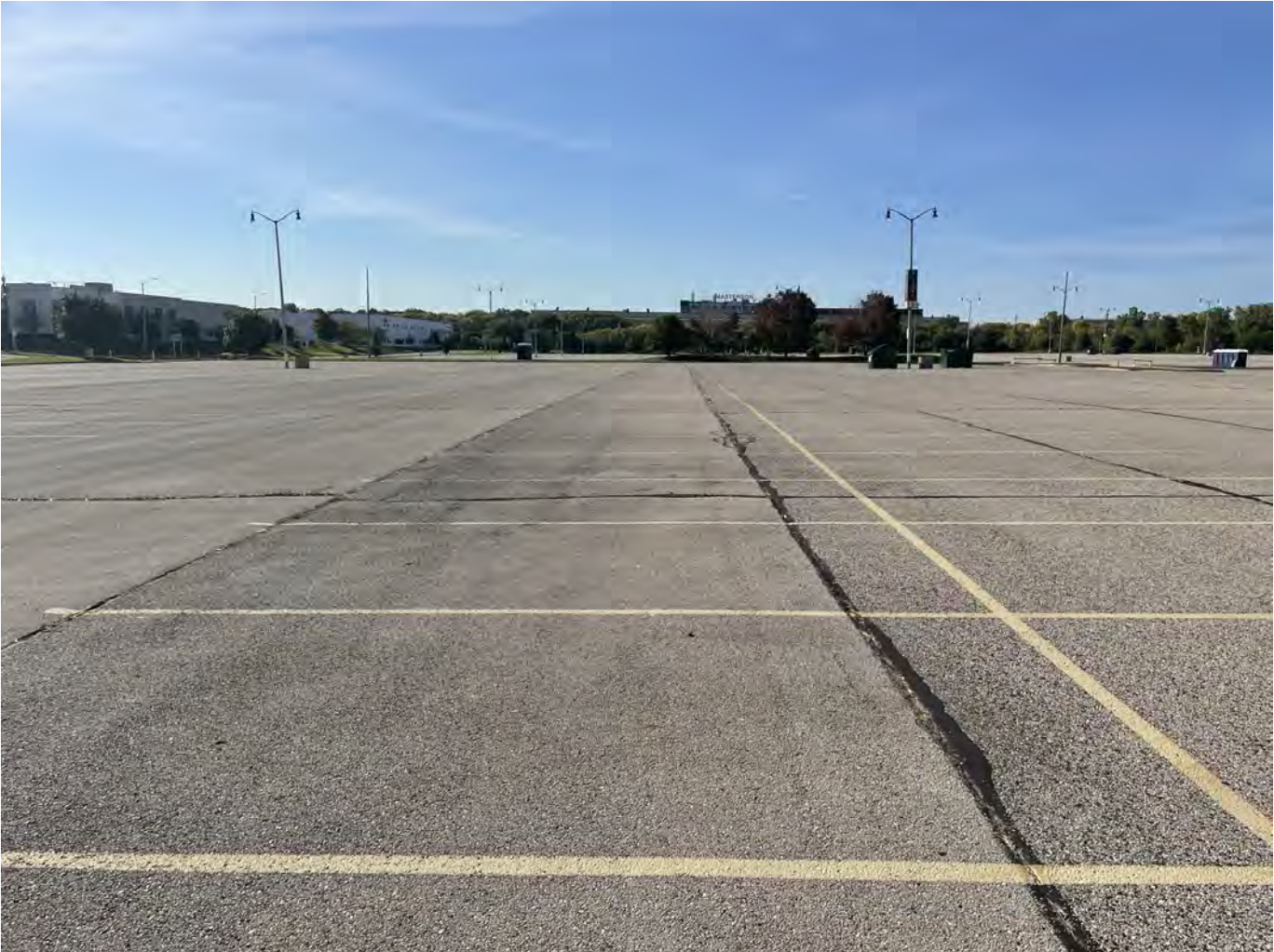
Photo 27: Yount Lot: Asphalt cap over Yount Lot: 4-inch asphalt pavement overlying 8-inches of crushed aggregate base course. Photo taken facing south on October 4, 2022.
