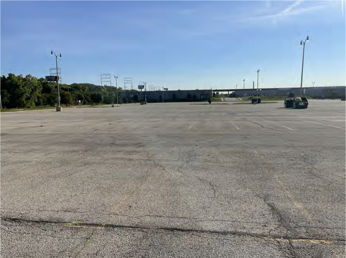
Photo 21: Yount Lot: Asphalt cap over Yount Lot: 4-inch asphalt pavement overlying 8-inches of crushed aggregate base course. Photo taken facing east on October 4, 2022.
