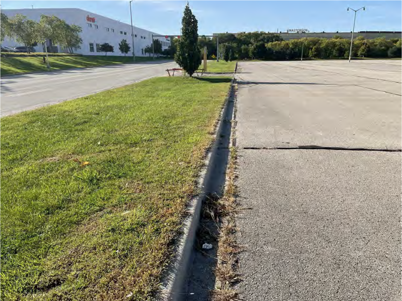
Photo 3: Yount Lot: Asphalt cap over Yount Lot (right side of photo): 4-inch asphalt pavement overlying 8-inches of crushed aggregate base course. Greenspace cap over parking lot median: 12-inches of low-permeability non-impacted soil covered with 4-inches of vegetated topsoil. Concrete curb and gutter along median perimeter and edge of asphalt pavement. Photo taken facing south on October 4, 2022.
