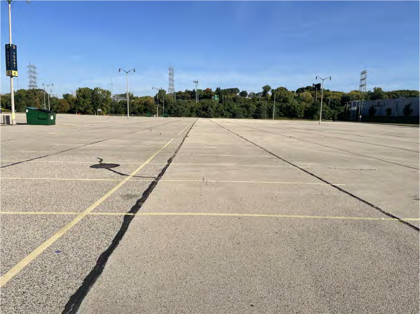
Photo 28: Yount Lot: Asphalt cap over Yount Lot: 4-inch asphalt pavement overlying 8-inches of crushed aggregate base course. Photo taken facing north on October 4, 2022.
