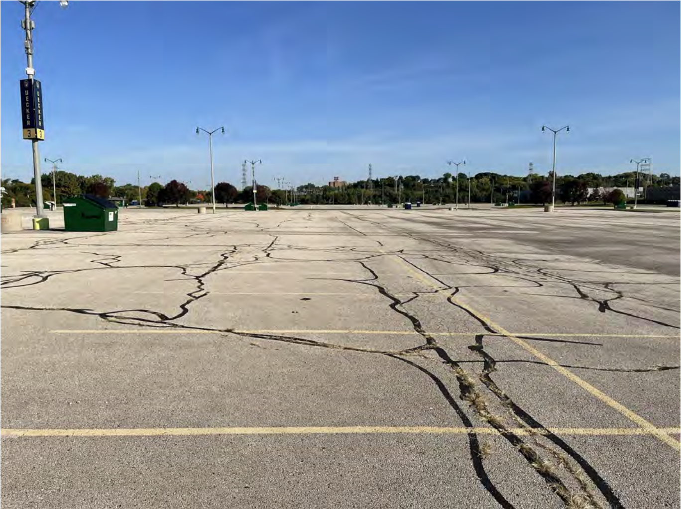
Photo 12: Uecker Lot: Asphalt cap over Uecker Lot: 4-inch asphalt pavement overlying 8-inches of crushed aggregate base course. Photo taken facing north on October 4, 2022.
