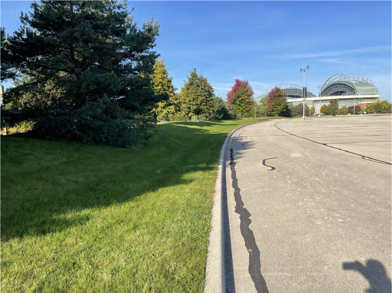
Photo 8: Uecker Lot: Asphalt cap over Uecker Lot (right side of photo): 4-inch asphalt pavement overlying 8-inches of crushed aggregate base course. Greenspace cap over parking lot median along Frederick Miller Way on south side of Uecker Lot: 12-inches of low-permeability non-impacted soil covered with 4-inches of vegetated topsoil. Concrete curb and gutter along median perimeter and edge of asphalt pavement. Photo taken facing west-northwest on October 4, 2022.
