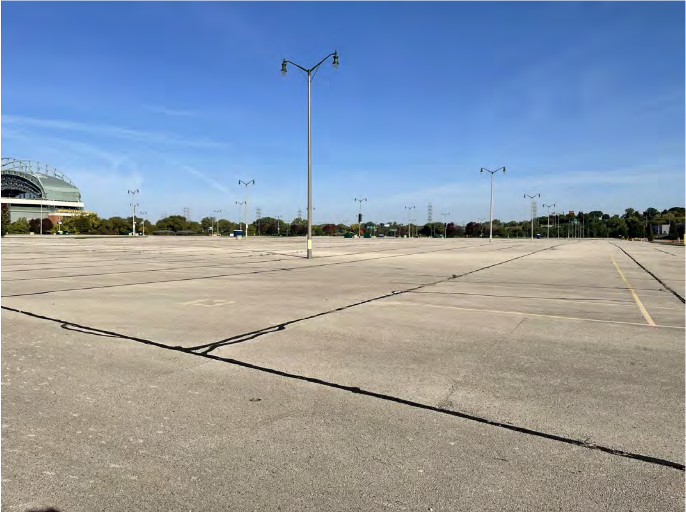
Photo 9: Uecker Lot: Asphalt cap over Uecker Lot: 4-inch asphalt pavement overlying 8-inches of crushed aggregate base course. Photo taken facing northwest on October 4, 2022.
