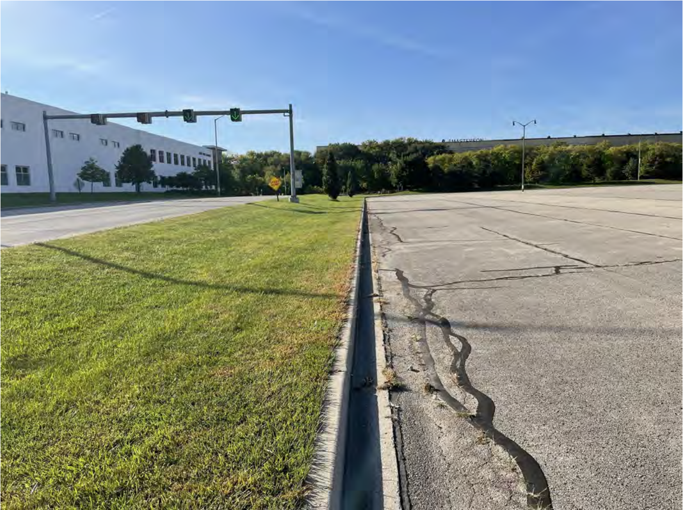
Photo 5: Uecker Lot: Asphalt cap over Uecker Lot (right side of photo): 4-inch asphalt pavement overlying 8-inches of crushed aggregate base course. Greenspace cap over parking lot median: 12-inches of low-permeability non-impacted soil covered with 4-inches of vegetated topsoil. Concrete curb and gutter along median perimeter and edge of asphalt pavement. Photo taken facing south on October 4, 2022.
