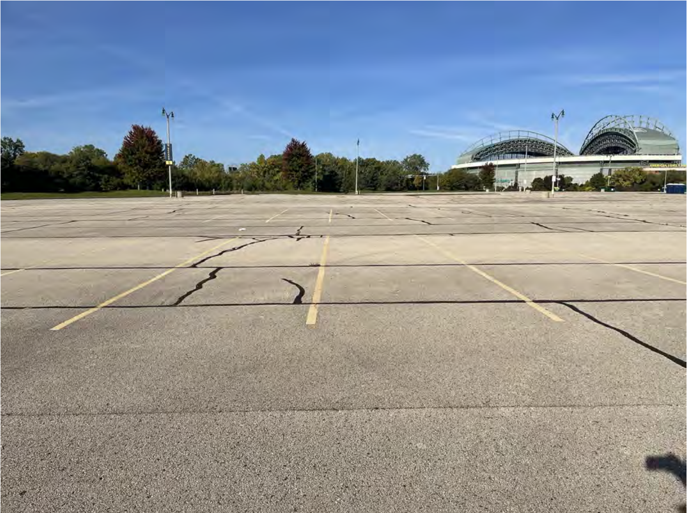
Photo 7: Uecker Lot: Asphalt cap over Uecker Lot: 4-inch asphalt pavement overlying 8-inches of crushed aggregate base course. Photo taken facing west on October 4, 2022.
