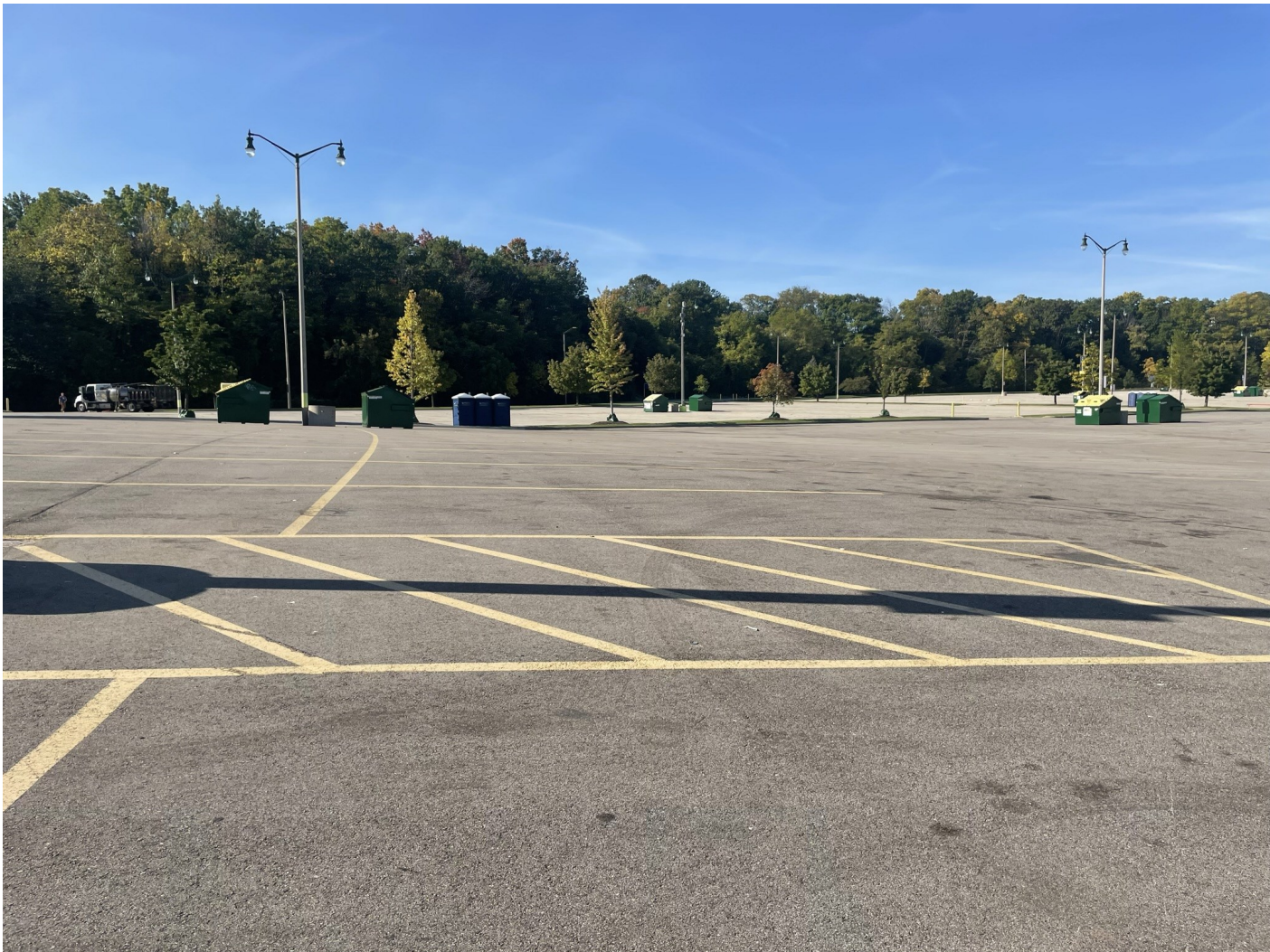
Photo 66: Aaron Lot: Asphalt cap surface lot: 4-inch asphalt pavement over 8-inches of crushed aggregate. Photo taken facing west on October 4, 2022.
