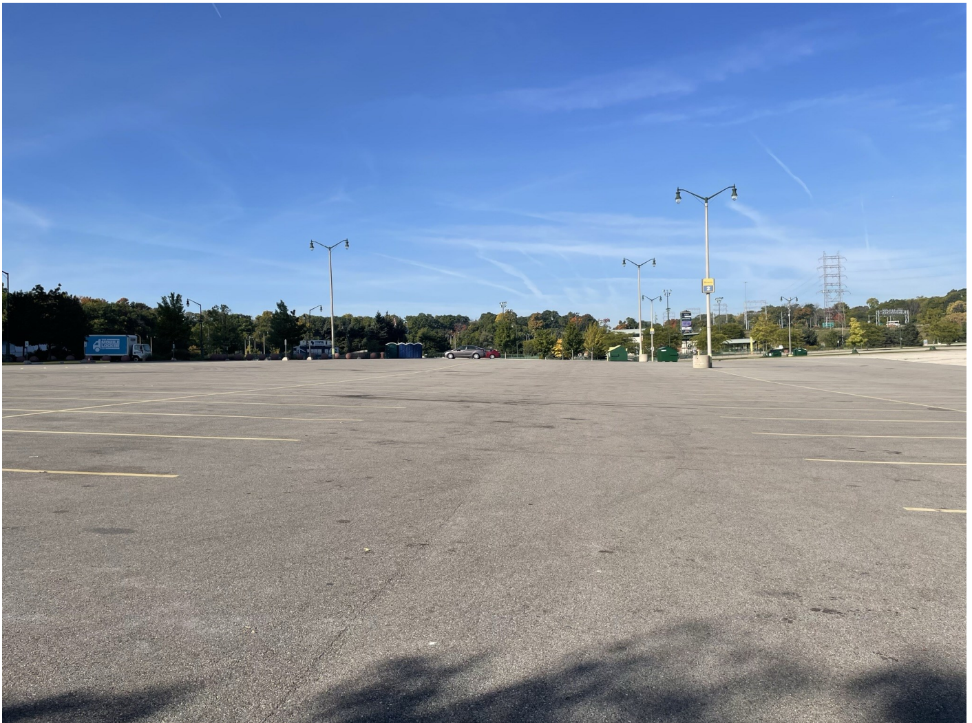
Photo 47: Brewers and Braves Lots plus Selig Drive: Brewers 2 Lot paved with asphalt surface cap: 4-inch asphalt pavement over 8-inches of crushed aggregate. No holes, major cracks, or other compromises. Photo taken facing west on October 4, 2022.
