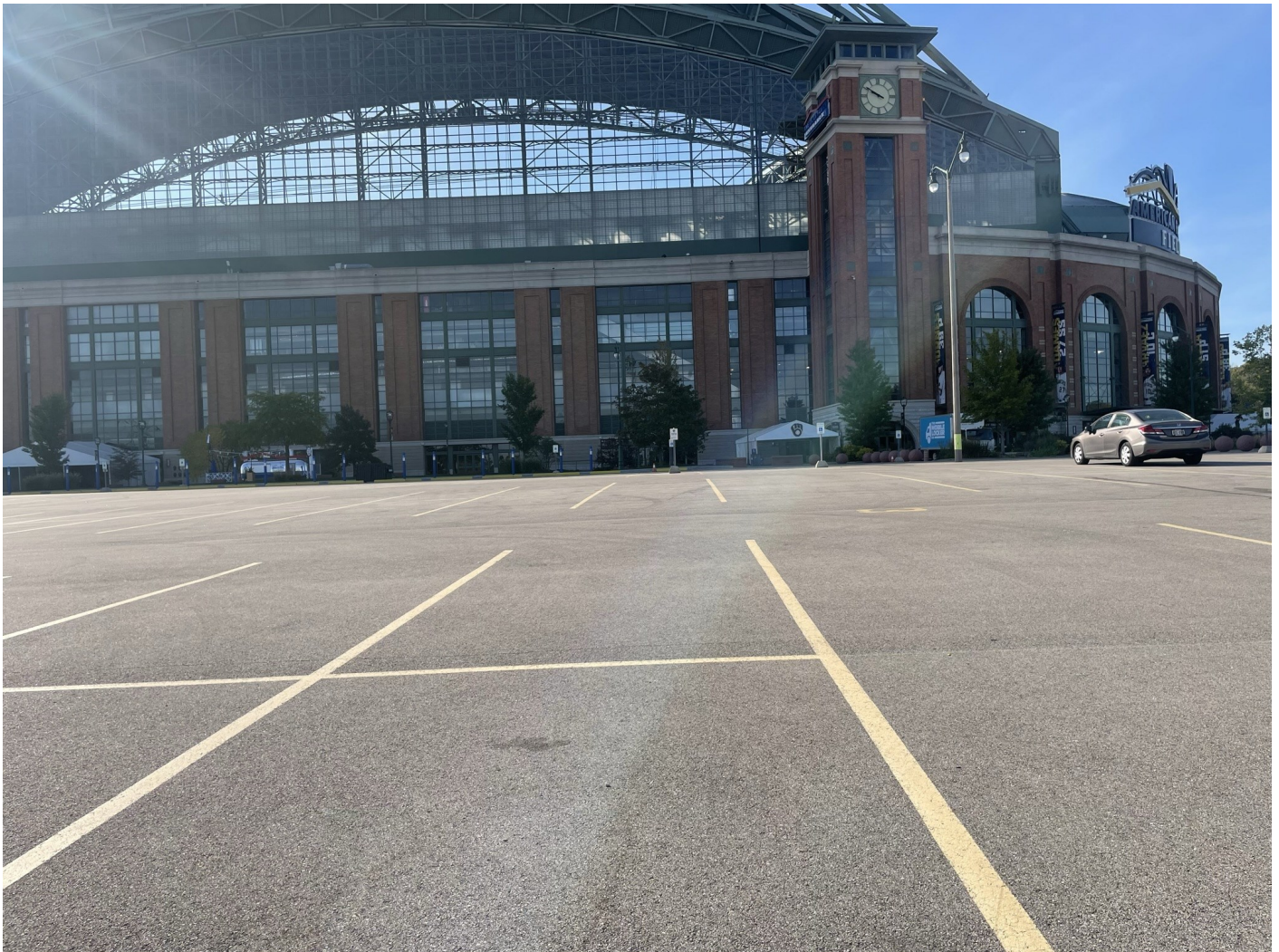
Photo 49: Brewers and Braves Lots plus Selig Drive: Brewers 2 Lot paved with asphalt surface cap: 4-inch asphalt pavement over 8-inches of crushed aggregate. No holes, major cracks, or other compromises. Photo taken facing south on October 4, 2022.
