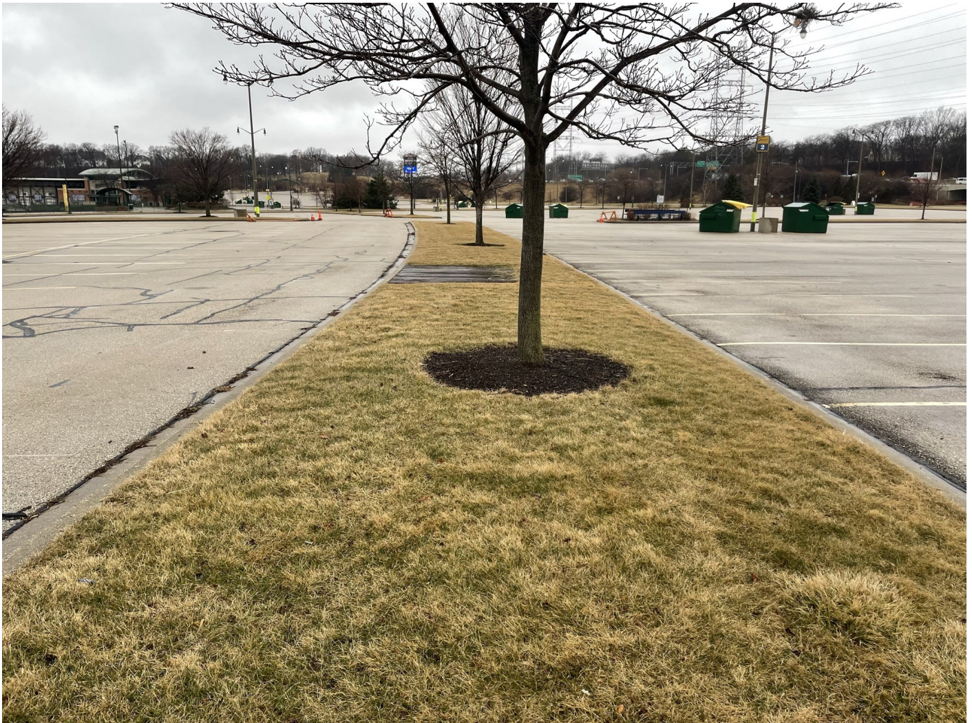
Photo 48: Brewers and Braves Lots plus Selig Drive: Brewers 2 Lot (left) and Braves 2 Lot (right) paved with asphalt surface cap: 4-inch asphalt pavement over 8-inches of crushed aggregate. No holes, major cracks, or other compromises. Landscaped median between each lot: Grass greenspace cap: grass topsoil over 12-inches of low permeability non-impacted soil. Photo taken facing west on January 18, 2023.
