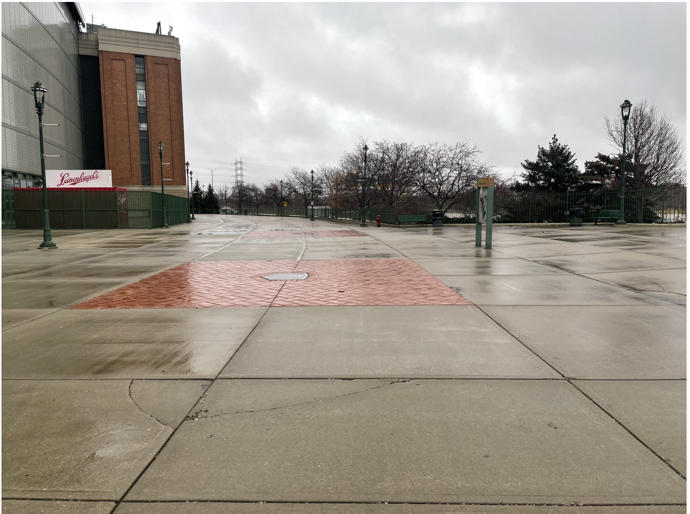
Photo 40: Stadium Plaza area (southeast side of stadium): Concrete pavement cap along exterior plaza sections and pedestrian sidewalk. 6-inches of concrete pavement over crushed aggregate. Decorative brick pavers within memorial sections of the plaza shown in central portion of the photo.
