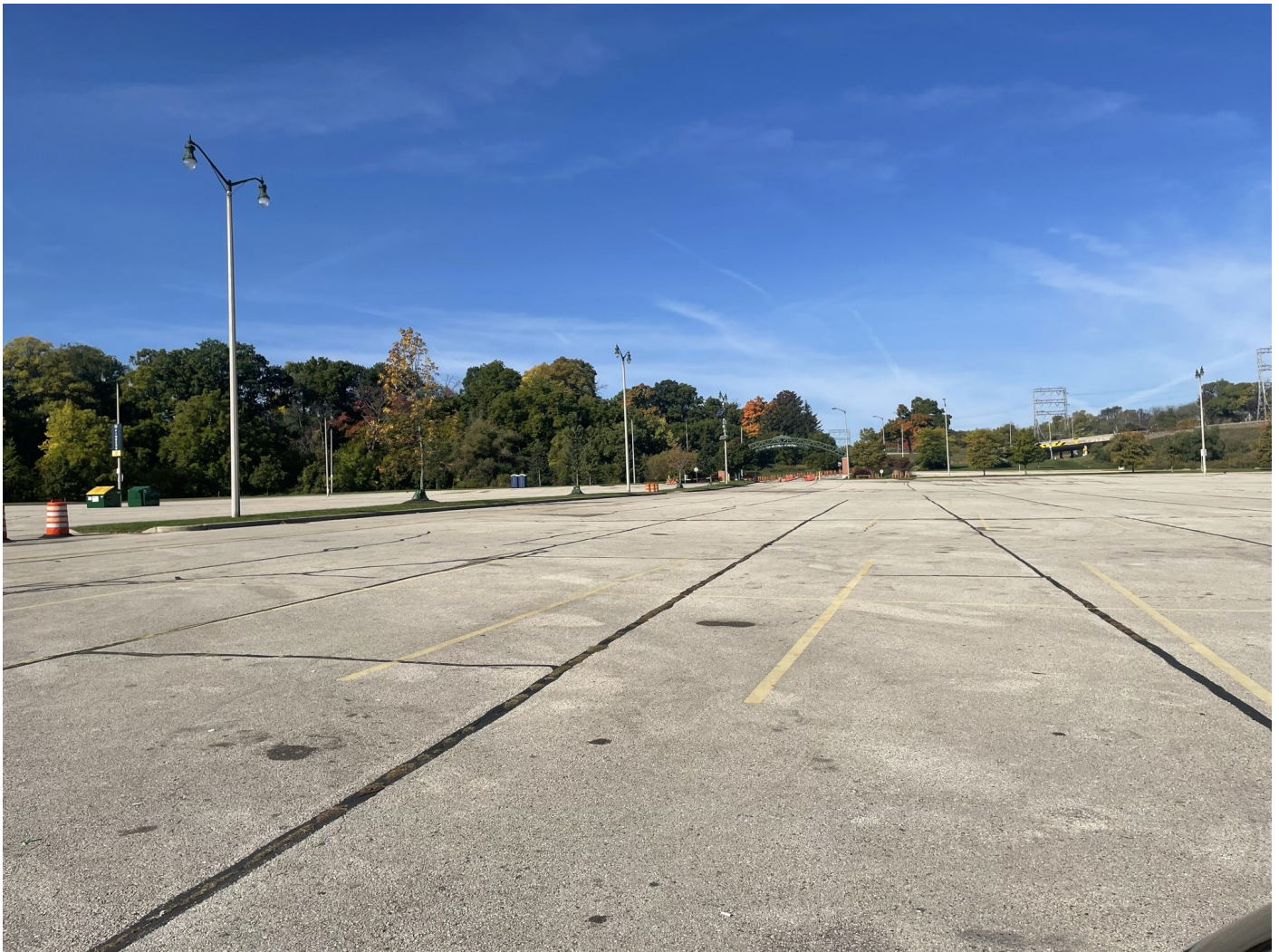
Photo 67: Money Lot: Asphalt cap surface lot: 4-inch asphalt pavement over 8-inches of crushed aggregate. Photo taken facing northwest on October 4, 2022.
