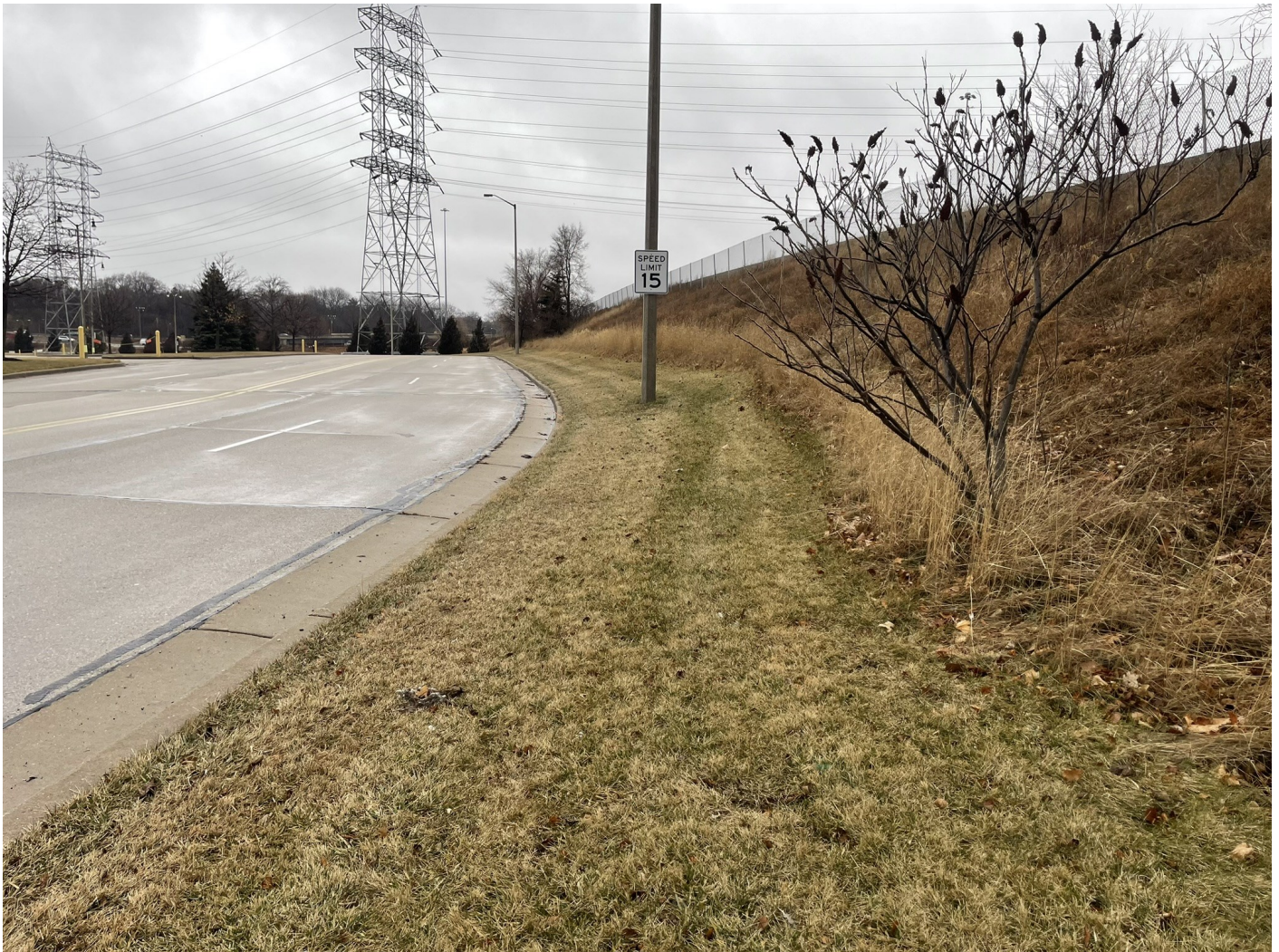
Photo 46: Brewers and Braves Lots plus Selig Drive: Greenspace landscaping along the east side of Selig Drive along Brewers and Braves Lots. Grass topsoil over 12-inches low permeability non-impacted soil. No ruts or holes in cap. Concrete curb and gutter cap, and asphalt pavement cap along roadway shown in left portion of photo. Photo taken facing northwest on January 18, 2023.
