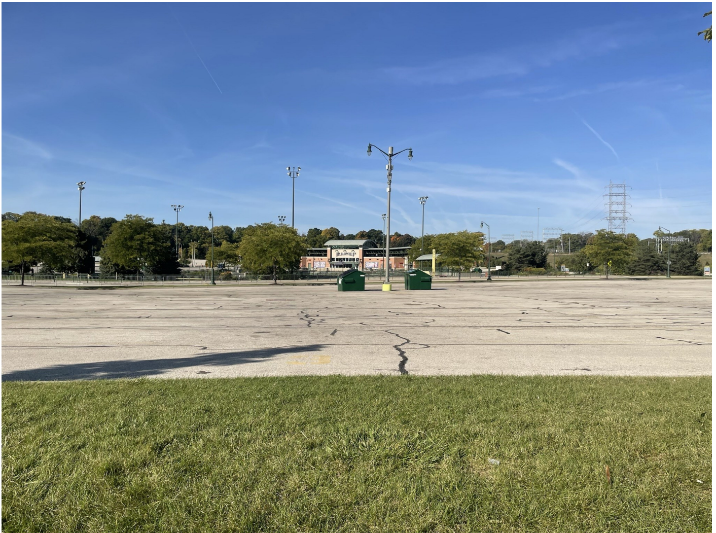
Photo 50: Brewers and Braves Lots plus Selig Drive: Brewers 1 Lot paved with asphalt surface cap: 4-inch asphalt pavement over 8-inches of crushed aggregate. Greenspace median cap shown in photo foreground. Photo taken facing west on October 4, 2022.
