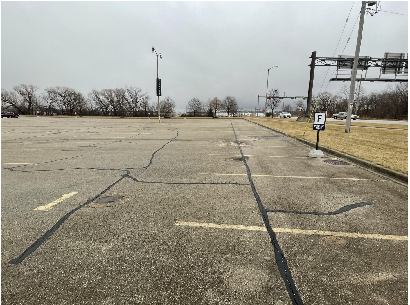
Photo 26: Ganter Lot: Asphalt cap across the entire Ganter Lot parking lot, representative of asphalt parking lot caps across the River West site. 4-inch asphalt pavement over 8-inches of crushed aggregate (base course). Photo taken facing east on January 18, 2023.
