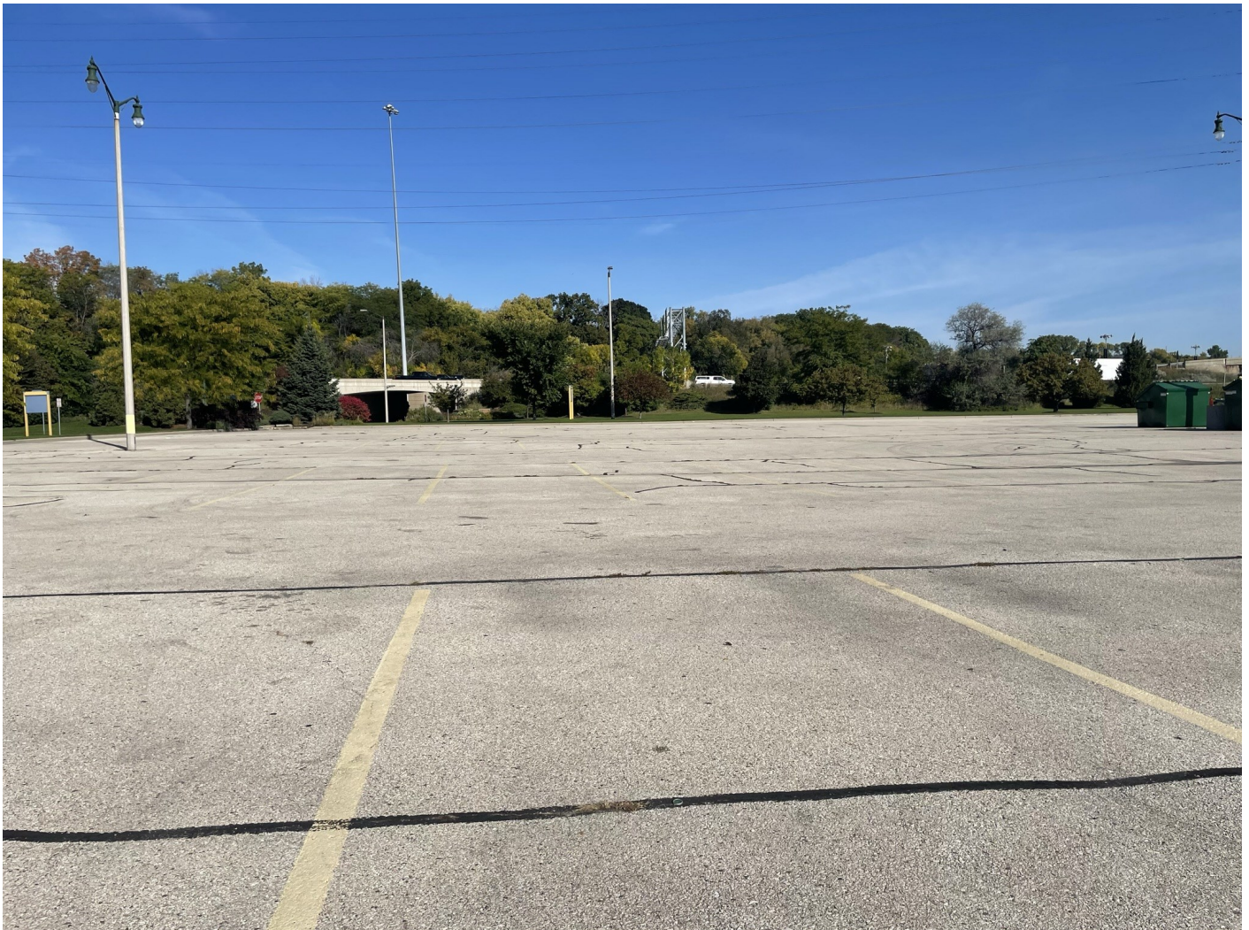
Photo 53: Brewers and Braves Lots plus Selig Drive: Braves 1 Lot paved with asphalt surface cap: 4-inch asphalt pavement over 8-inches of crushed aggregate. Photo taken facing north on October 4, 2022.
