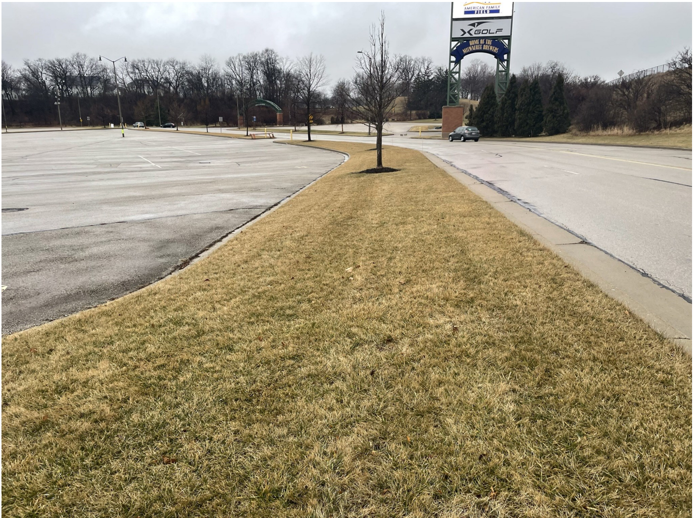
Photo 64: Money Lot: Asphalt cap surface lot: 4-inch asphalt pavement over 8-inches of crushed aggregate shown in left portion of photo. Greenspace cap median along northern edge of Money Lot, along south side of Selig Drive: 12-inches of low permeability soil covered with 4-inches of vegetated (grass) topsoil. Photo taken facing west on January 18, 2023.
