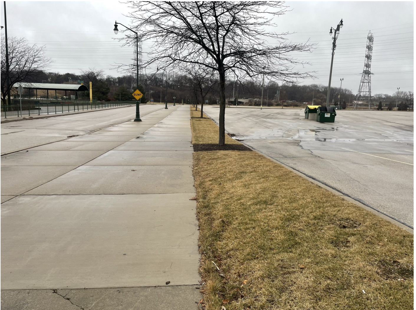
Photo 52: Brewers and Braves Lots plus Selig Drive: Asphalt cap entrance drive (left) along west side of Brewers 1 Lot. Concrete cap sidewalk along west side of Brewers 1 Lot. Greenspace cap median along west side of Brewers 1 Lot. Photo taken facing north on January 18, 2023.
