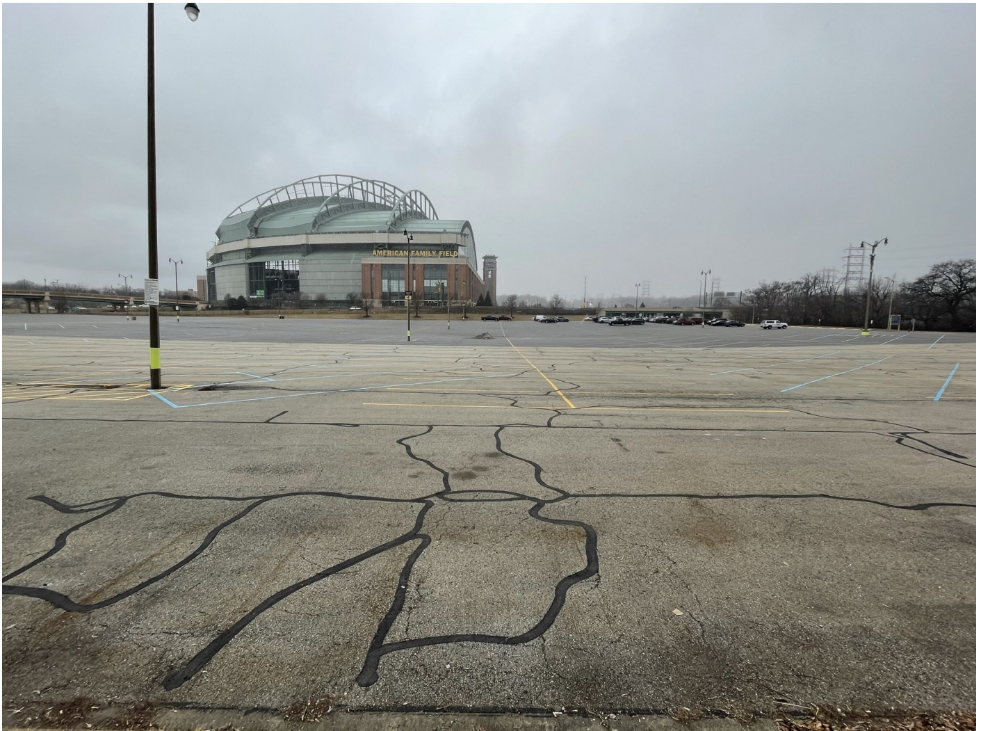
Photo 18: American Family Lot: Asphalt capped surface parking lot (American Family Lot). 4-inches of asphalt pavement over 8-inches of crushed aggregate. Older asphalt shown on in photo foreground, patched along cracks with asphalt tar. Newer asphalt shown in photo background.
