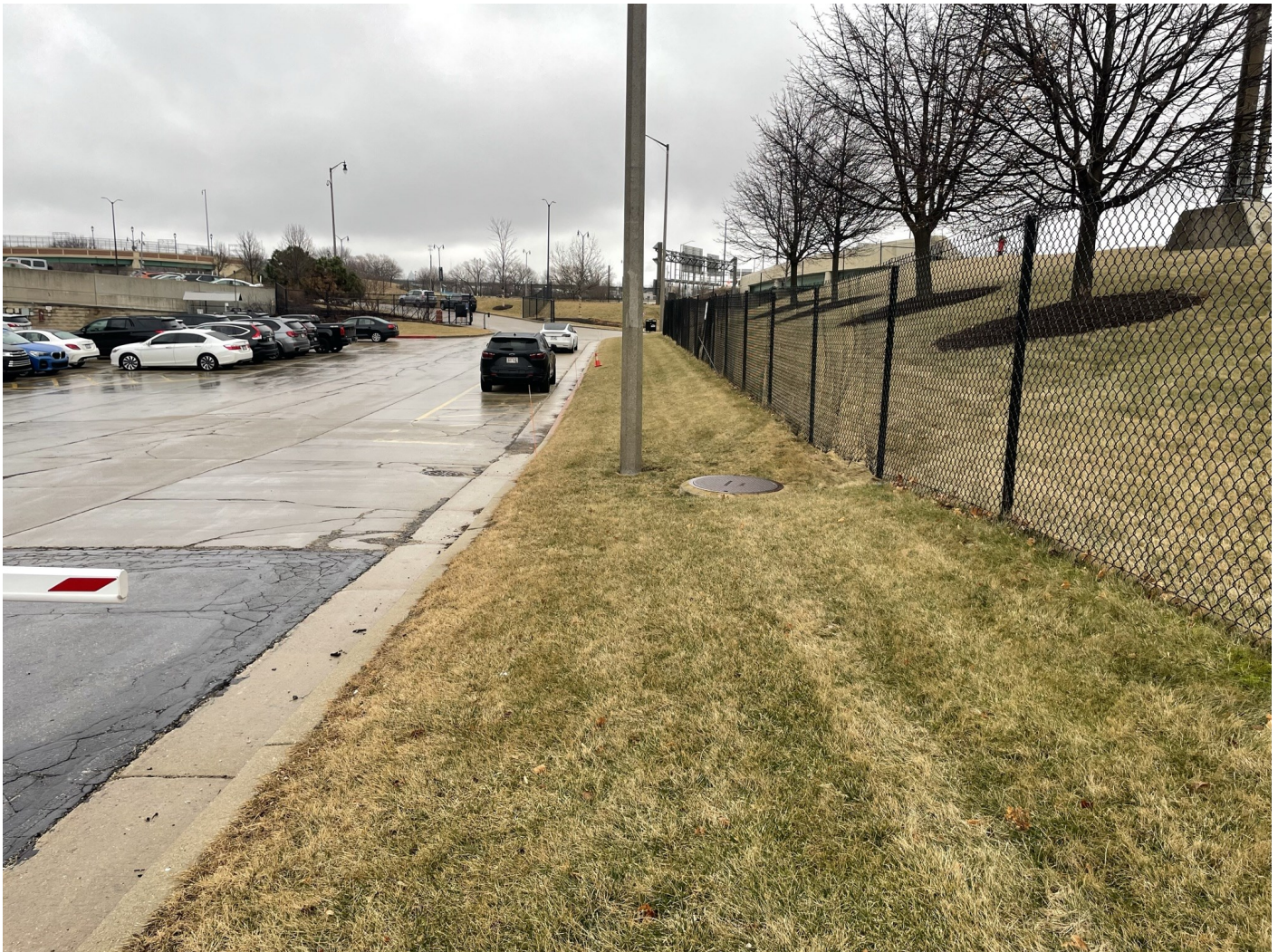
Photo 35: South Dock: Transition of asphalt pavement cap across Brewers Offices staff parking lot into concrete pavement South Dock area shown on left side of photo. Asphalt pavement is 4-inch asphalt over 8 inches crushed aggregate. Concrete loading dock pavement is 8-inch thick concrete over 8-inches crushed aggregate. Greenspace cap shown in central and right side portions of the photo: 12-inches low permeability non-impacted soil covered with vegetated (grass) topsoil. Photo taken facing east on January 18, 2023.
