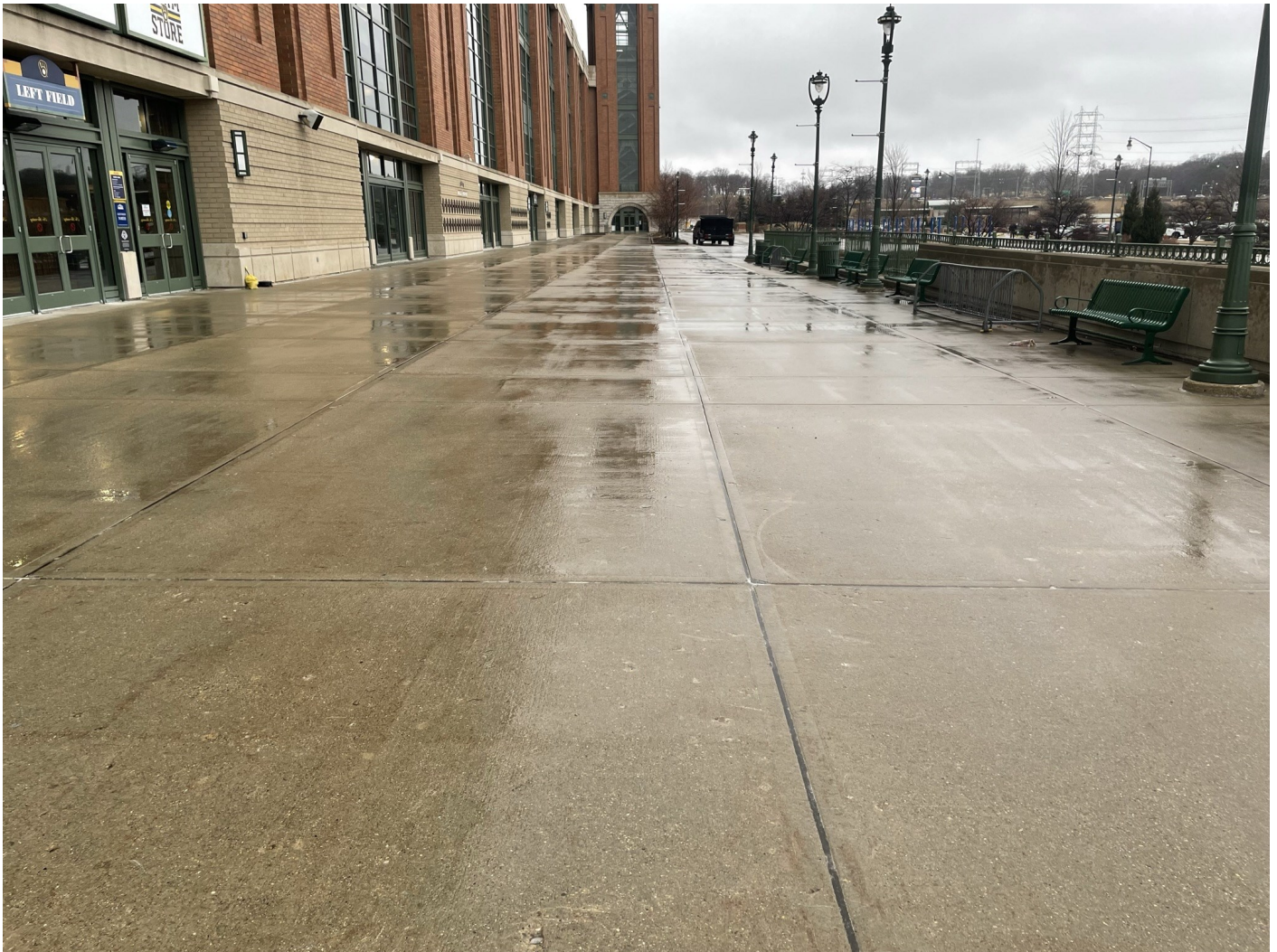
Photo 41: Stadium Plaza area (northeast side of stadium): Concrete pavement cap along exterior plaza sections and pedestrian sidewalk. 6-inches of concrete pavement over crushed aggregate. Photo taken facing west on January 18, 2023.
