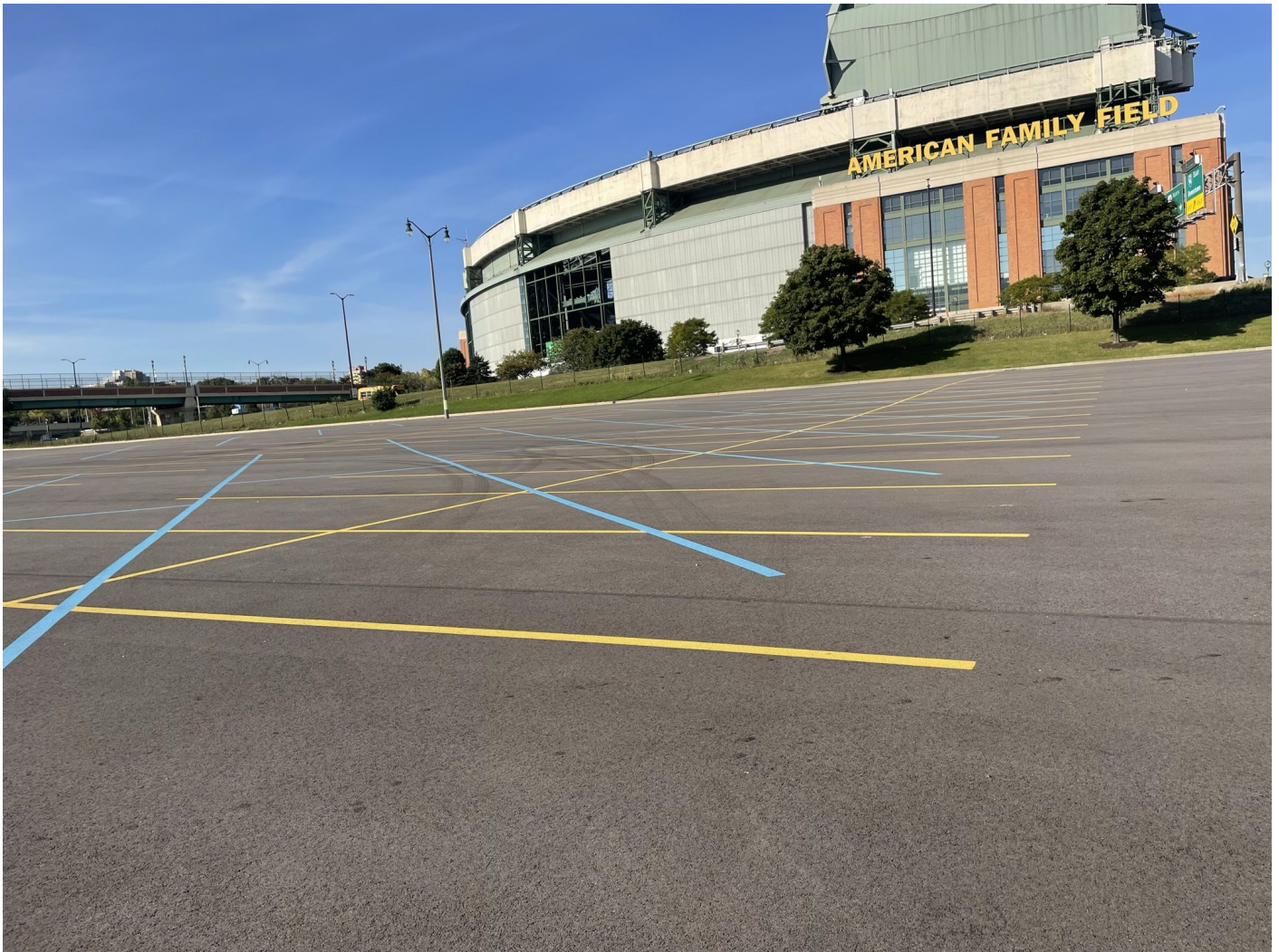
Photo 16: American Family Lot: Asphalt capped surface parking lot (American Family Lot). 4-inches of asphalt pavement over 8-inches of crushed aggregate. Photo taken facing southwest on October 4, 2022.
