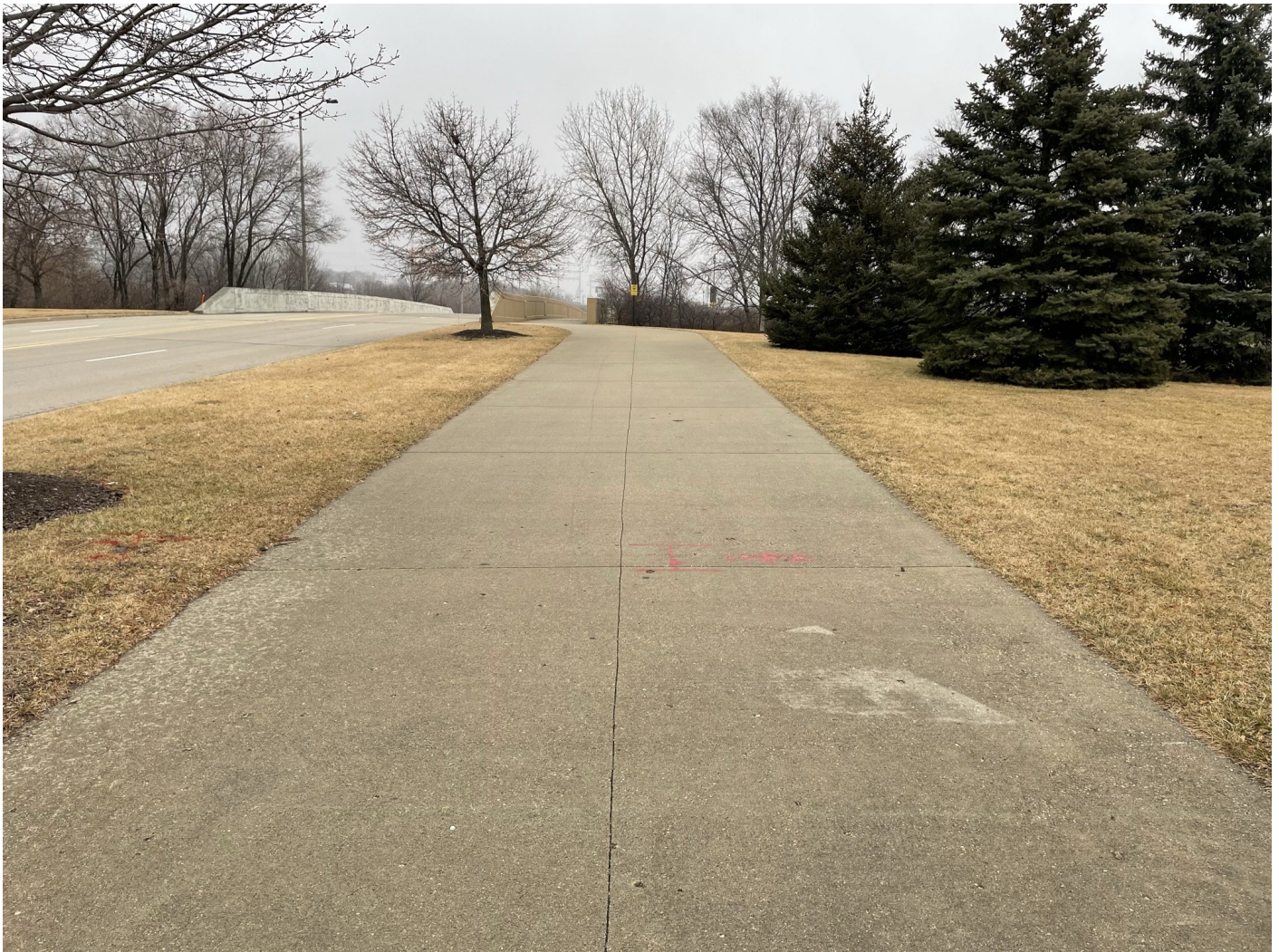
Photo 14: American Family Lot: Concrete pedestrian path cap along northern edge of the lot. 6-inches of concrete pavement over 8-inches of crushed aggregate. Greenspace cap shown on left and right side of photo. Photo taken facing east on January 18, 2023.
