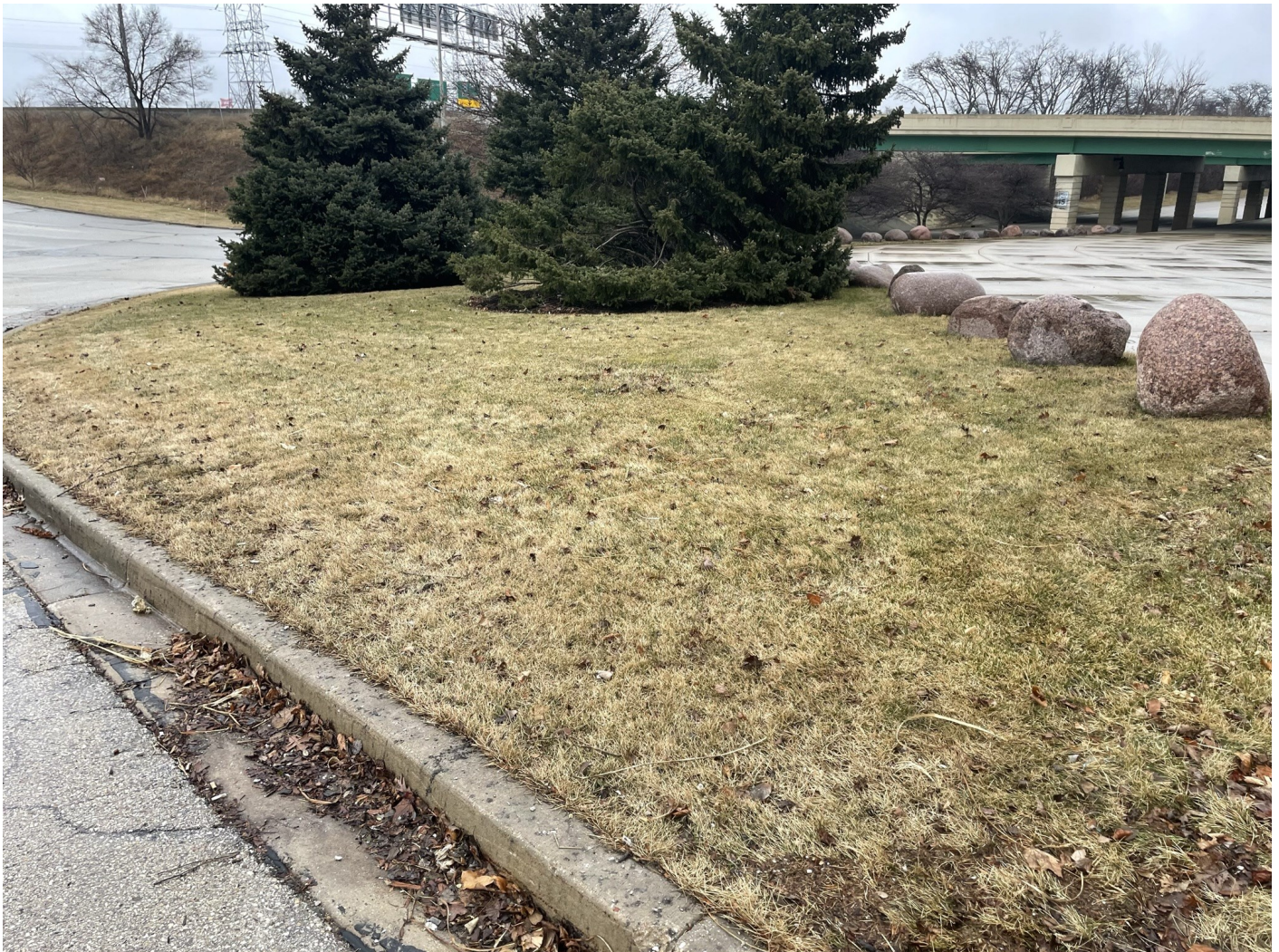
Photo 45: Brewers and Braves Lots plus Selig Drive: Greenspace landscaping with trees. Grass topsoil over 12-inches low permeability non-impacted soil. No ruts or holes in cap. Concrete curb and gutter cap shown in lower lefthand portion of photo. Photo taken facing northeast on January 18, 2023.
