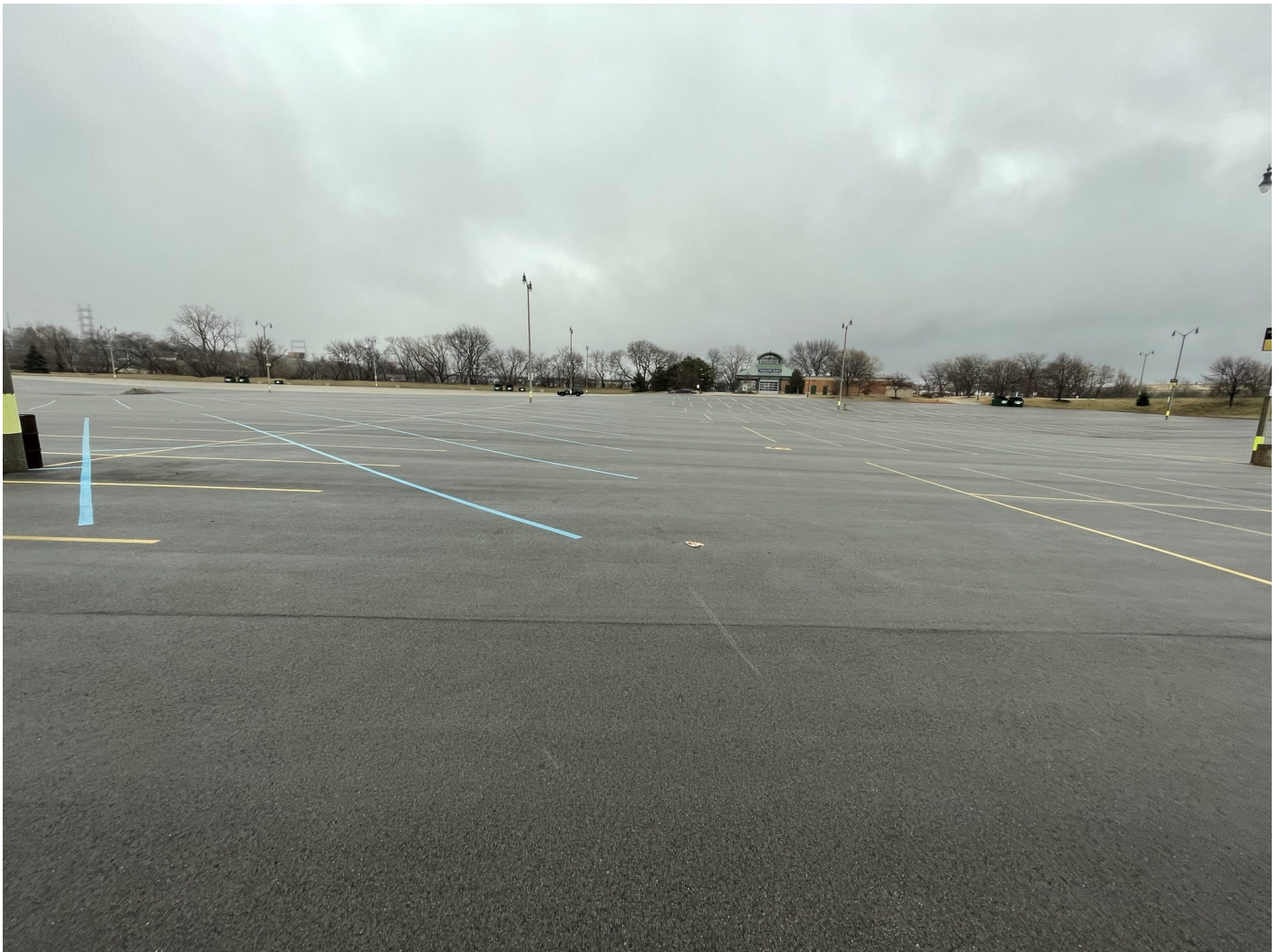
Photo 22: American Family Lot: Asphalt capped surface parking lot (American Family Lot). 4-inches of asphalt pavement over 8-inches of crushed aggregate. Photo taken facing east on January 18, 2023.
