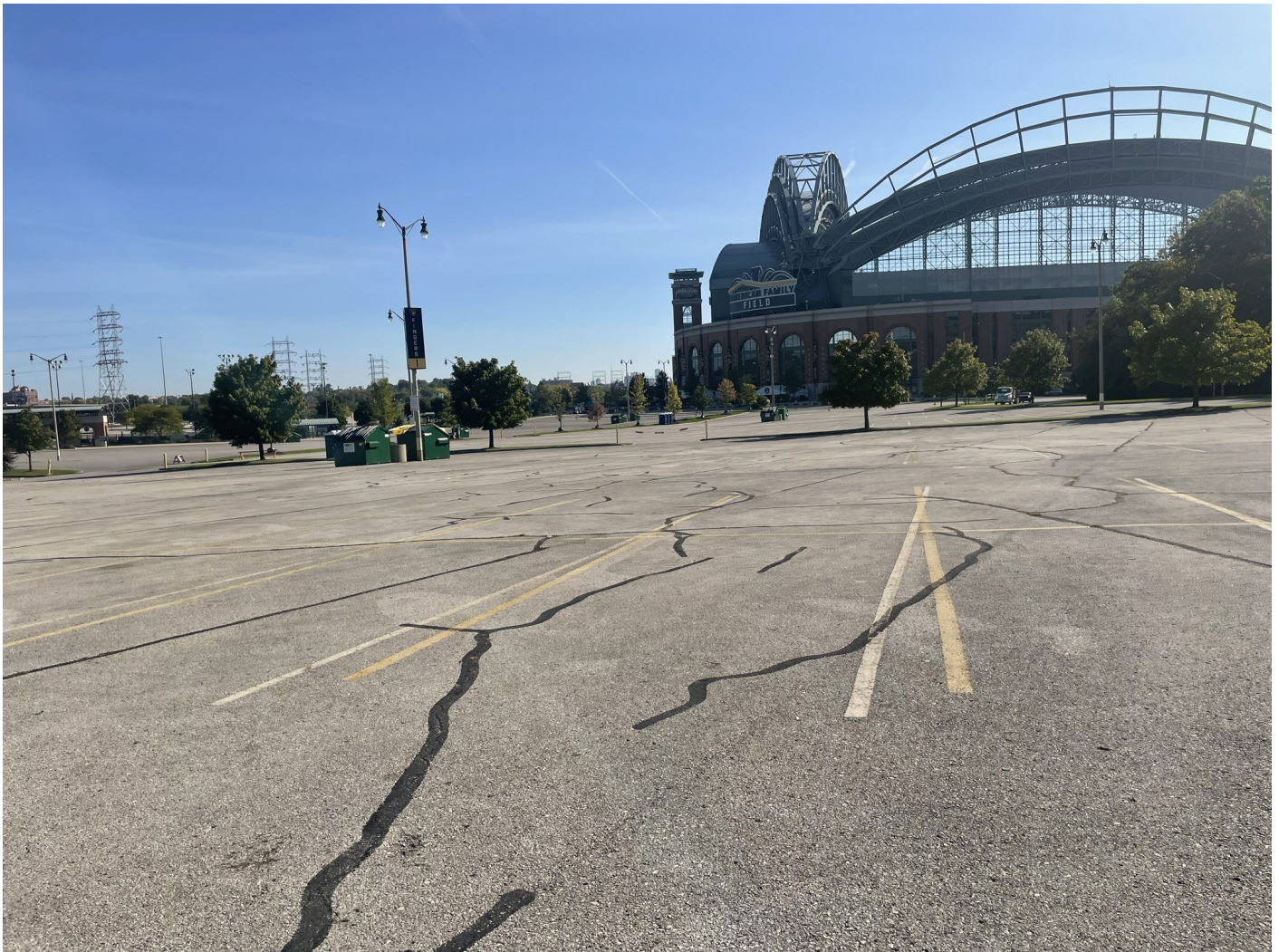
Photo 69: Fingers Lot: Asphalt cap surface lot: 4-inch asphalt pavement over 8-inches of crushed aggregate. Photo taken facing southeast on October 4, 2022.
