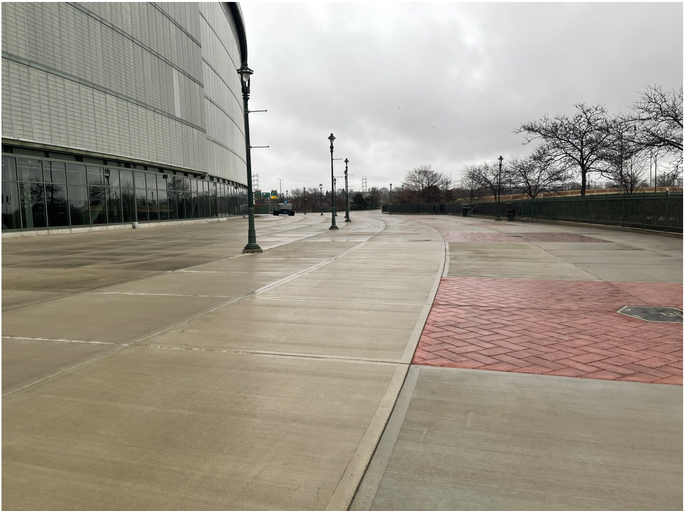
Photo 38: Stadium Plaza area (south side of stadium): Concrete pavement cap along exterior plaza sections and pedestrian sidewalk. 6-inches of concrete pavement over crushed aggregate. Decorative brick pavers within memorial sections of the plaza shown on the right side of the photo.
