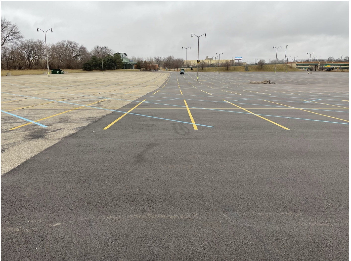
Photo 15: American Family Lot: Asphalt capped surface parking lot (American Family Lot). 4-inches of asphalt pavement over 8-inches of crushed aggregate. Older asphalt shown on left side of photo. Newer asphalt shown on right side of photo. Photo taken facing south on January 18, 2023.
