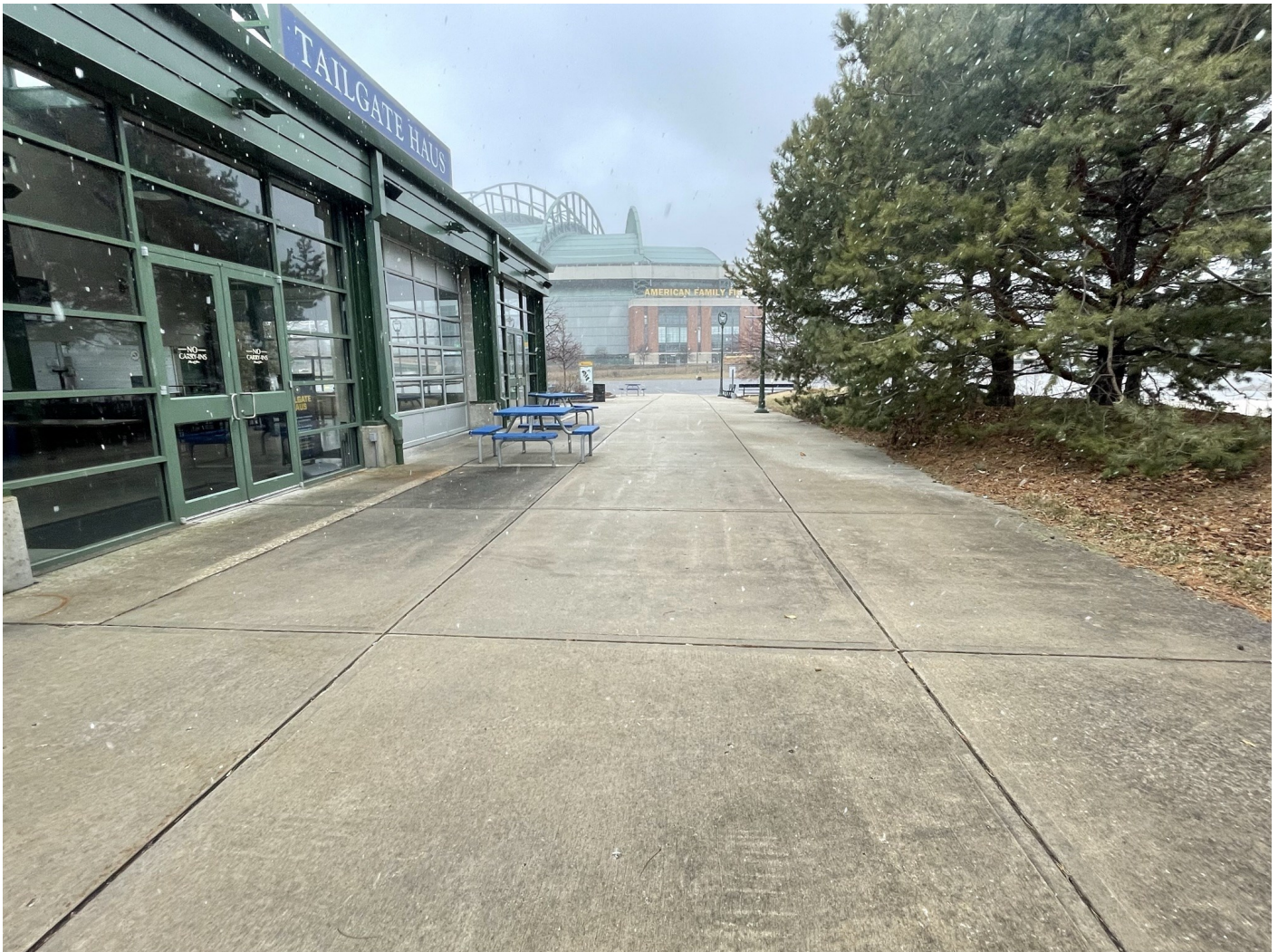
Photo 19: American Family Lot: Concrete pavement plaza area / pedestrian walk along north side of Tailgate Haus in the American Family Lot. 6-inches of concrete over 8-inches crushed aggregate. Tailgate Haus with concrete floor slab/foundation shown on left side of photo. Landscaped berm (greenspace cap) shown on right side of photo. Photo taken facing west on January 18, 2023.
