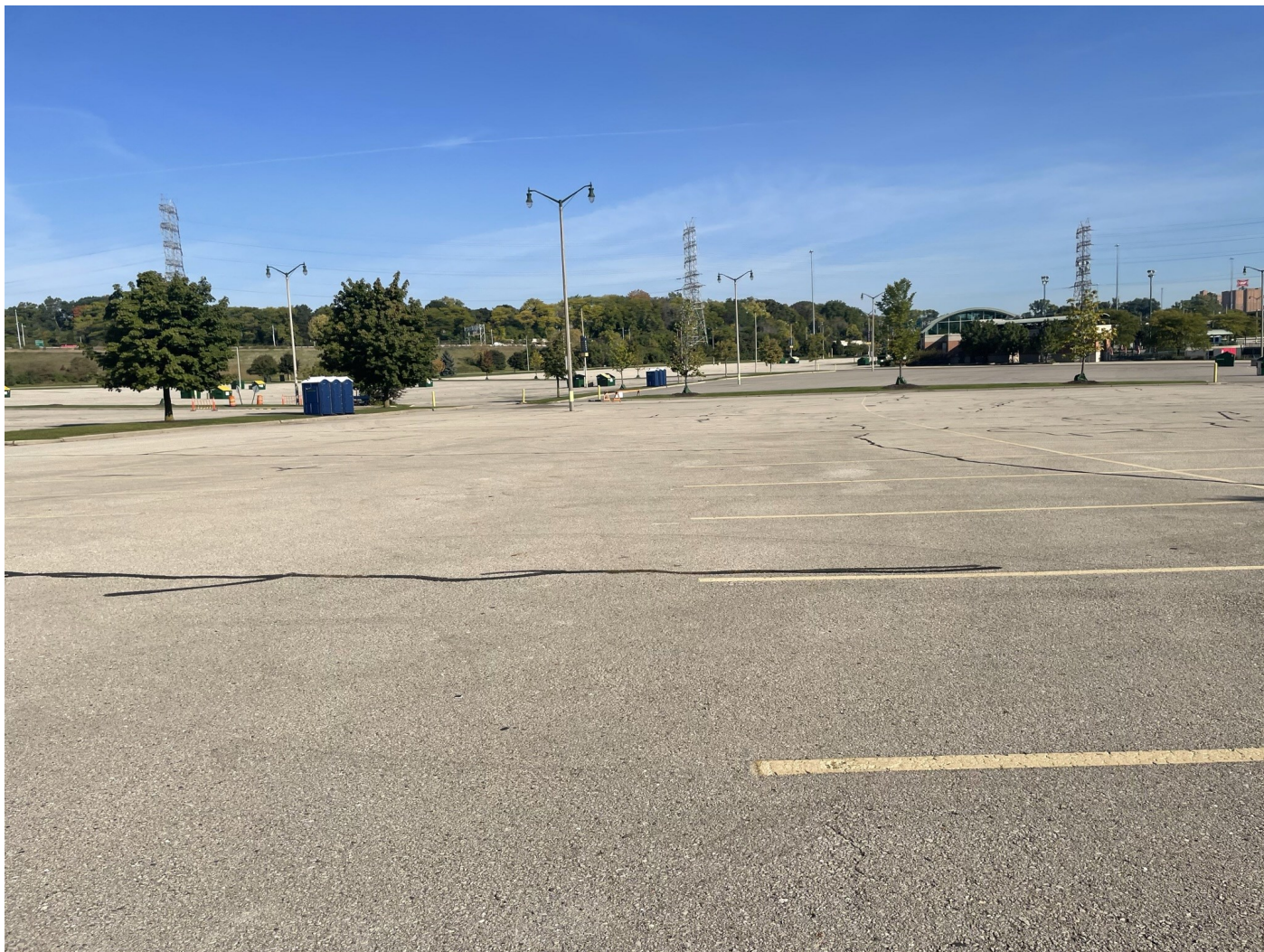
Photo 73: Thomas Lot: Asphalt cap surface lot: 4-inch asphalt pavement over 8-inches of crushed aggregate. Photo taken facing northeast on October 4, 2022.
