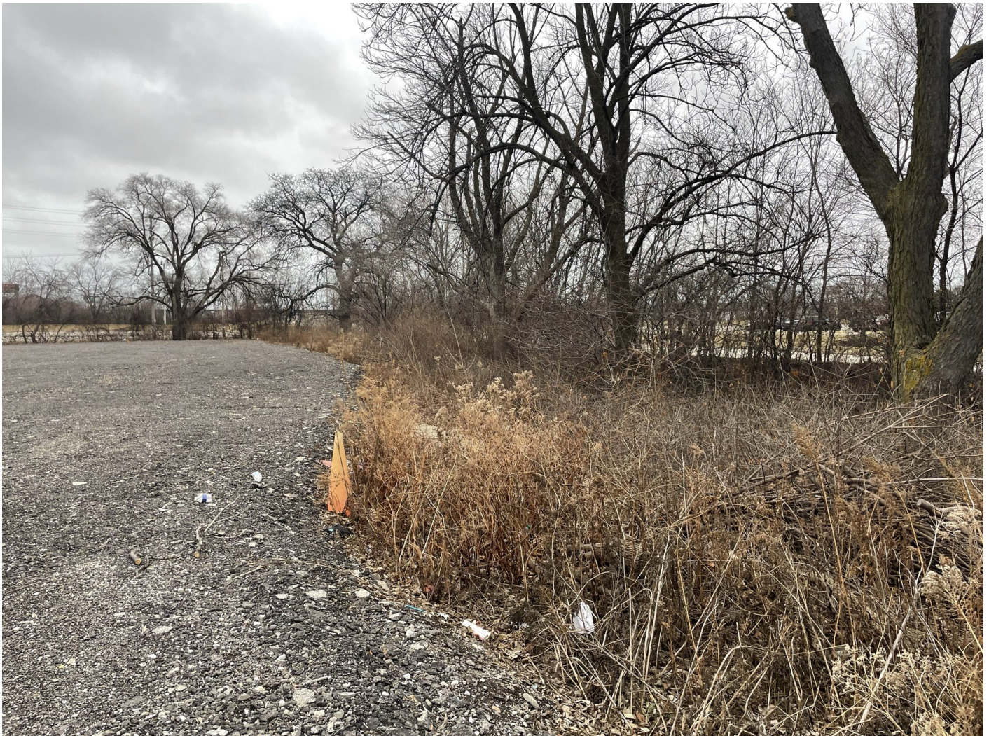
Photo 7: Staff Lot: Compacted milled asphalt cap across the Staff Lot. Between 6 and 12 inches thick. Overgrown vegetation and topsoil along perimeter, within perimeter fence. Photo taken facing east on January 18, 2023.
