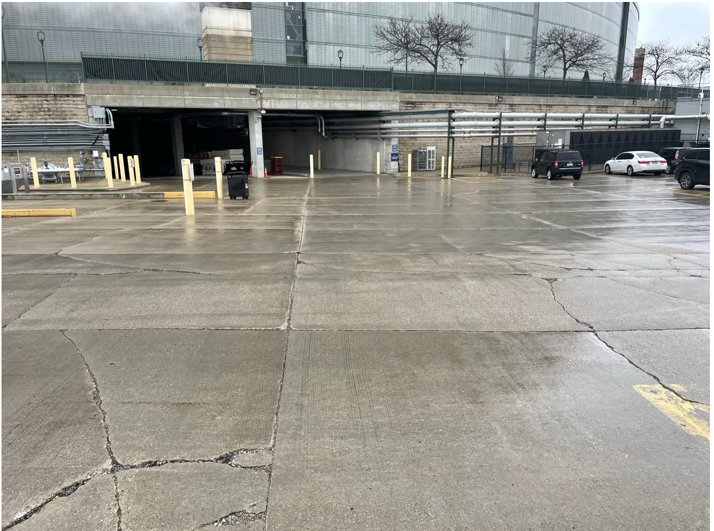
Photo 36: South Dock: Concrete loading dock pavement is 8-inch thick concrete over 8-inches crushed aggregate. Photo taken facing north on January 18, 2023.
