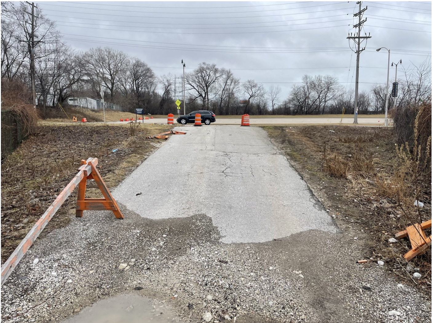
Photo 8: Staff Lot: Entrance driveway to the Staff Lot paved with asphalt (cap). Adjacent greenspace cap on each side of driveway. Photo taken facing east on January 18, 2023.
