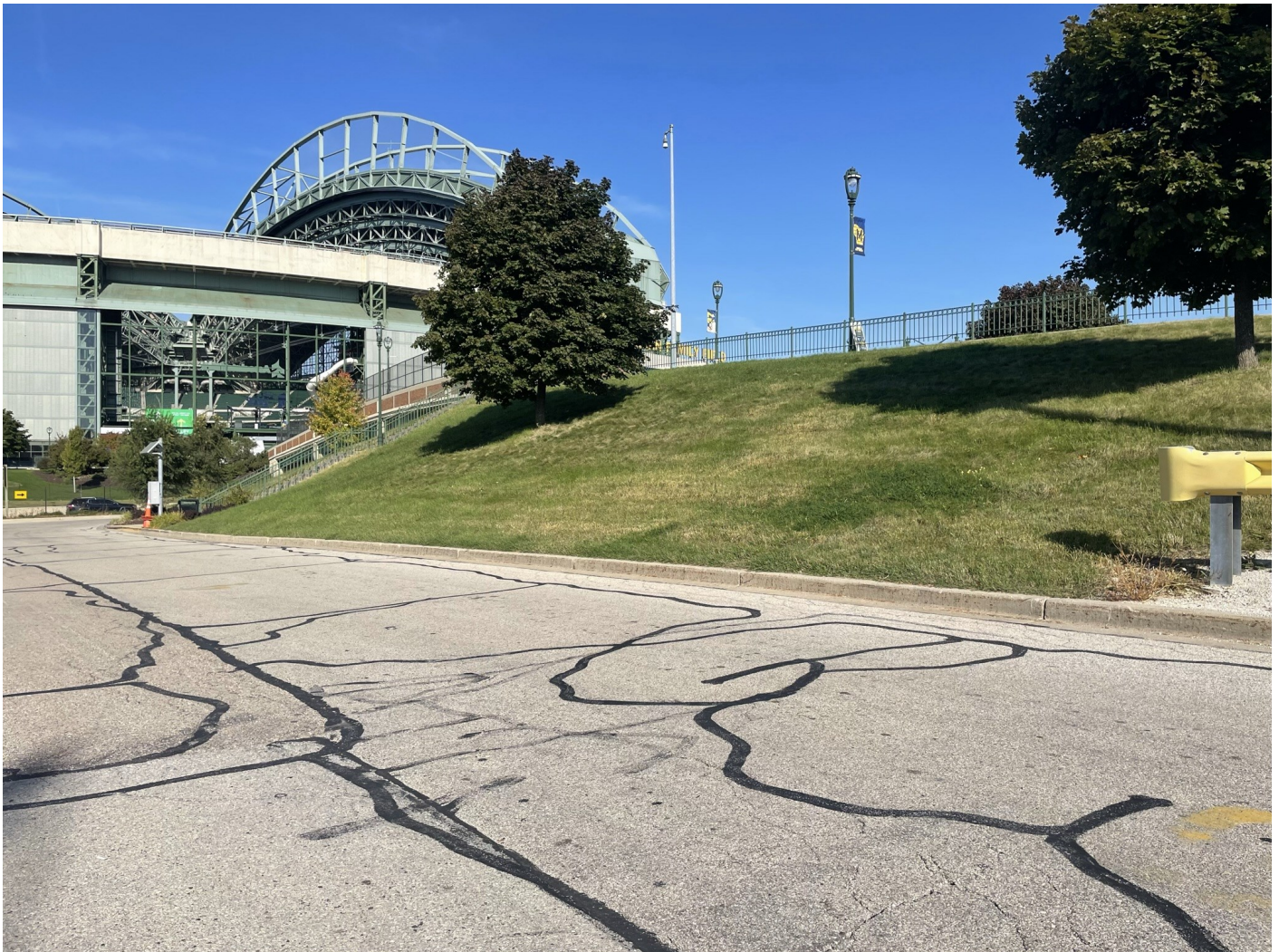
Photo 27: Kuenn Lot: Asphalt cap across Kuenn Lot parking lot, representative of asphalt parking lot caps across the River West site. 4-inch asphalt pavement over 8-inches of crushed aggregate. Concrete curb (6-inch thick concrete) and gutter (8-inch thick concrete) over crushed aggregate. Greenspace cap shown on right side of photo: 12-inches of low-permeability non-impacted soil covered with vegetated (grass) topsoil. Photo taken facing northwest on October 4, 2022.
