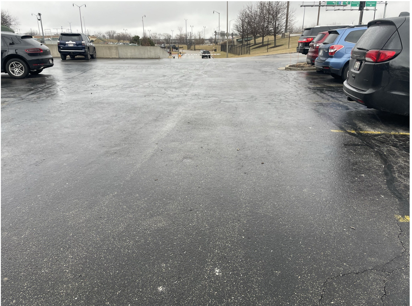
Photo 34: Brewers Offices Lot: Asphalt cap across Brewers Offices staff parking lot, representative of asphalt parking lot caps across the River West site. 4-inch asphalt pavement over 8-inches of crushed aggregate. Photo taken facing east on January 18, 2023.
