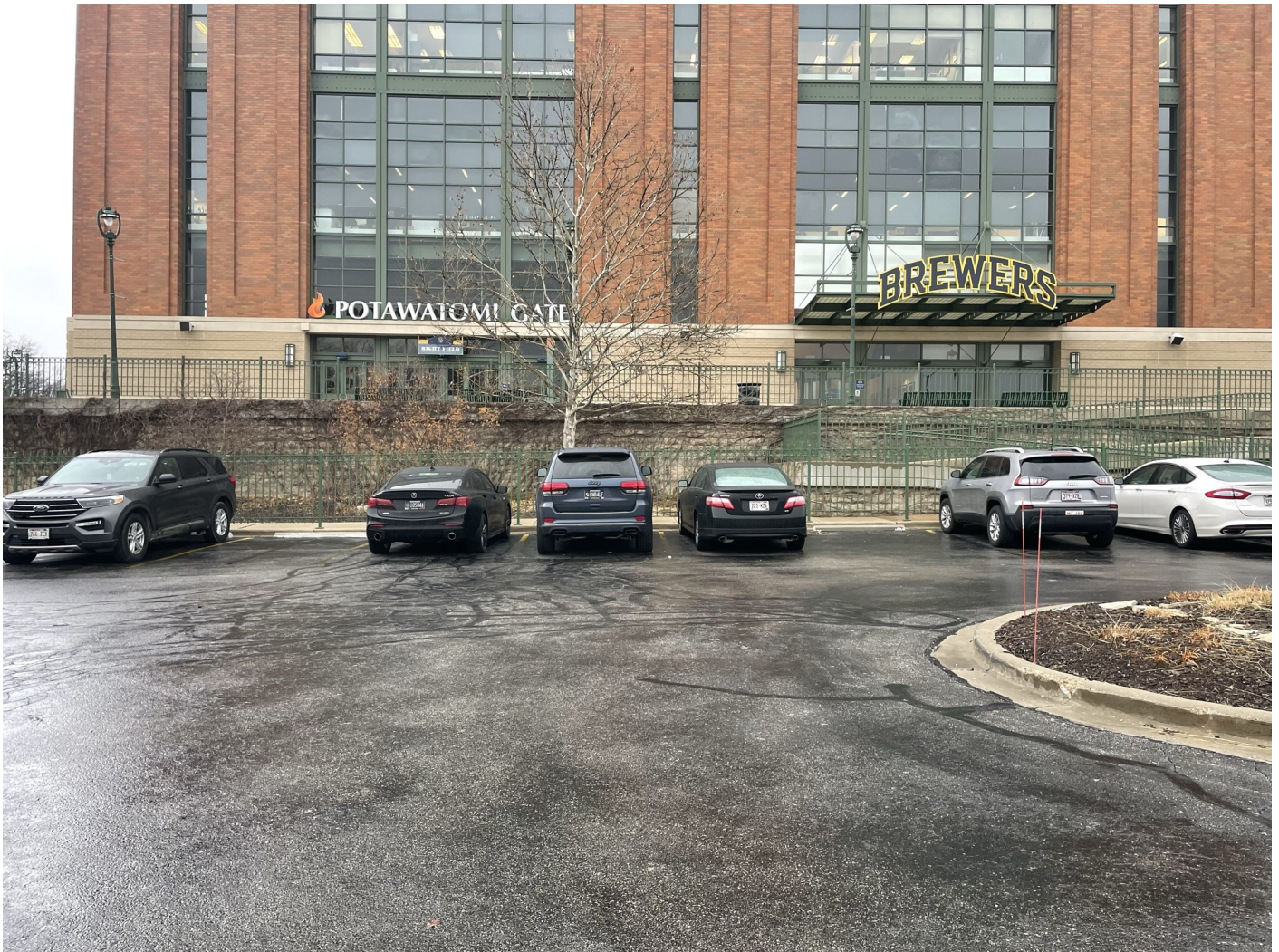
Photo 33: Brewers Offices Lot: Asphalt cap across Brewers Offices staff parking lot, representative of asphalt parking lot caps across the River West site. 4-inch asphalt pavement over 8-inches of crushed aggregate. Concrete curb (6-inch thick concrete) and gutter (8-inch thick concrete) over crushed aggregate shown on right side of photo. Greenspace cap within parking lot island shown on right side of photo: 12-inches of low-permeability non-impacted soil covered with mulched landscaping. Photo taken facing north on January 18, 2023.
