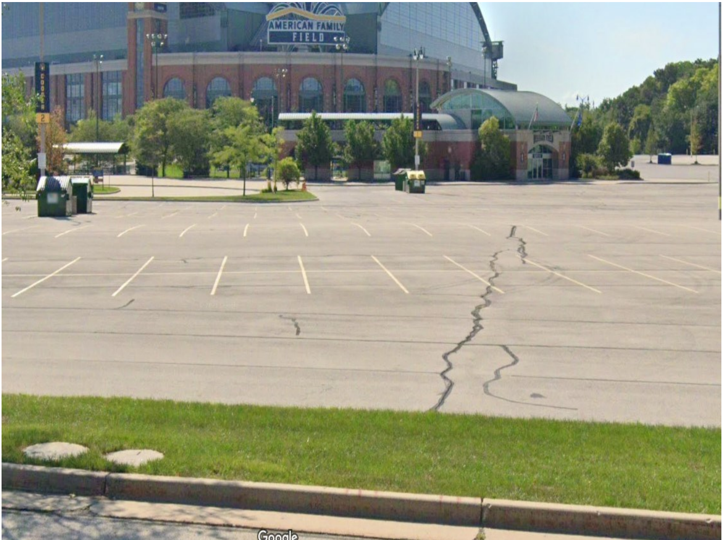
Photo 61: Cooper Lot area: Asphalt cap parking lot: 4-inch asphalt pavement cap over 8-inches of crushed aggregate base course. Greenspace median cap in photo foreground: 12-inches of low permeability non-impacted soil covered with 4-inches of vegetated topsoil. Photo taken facing south August 2021.
