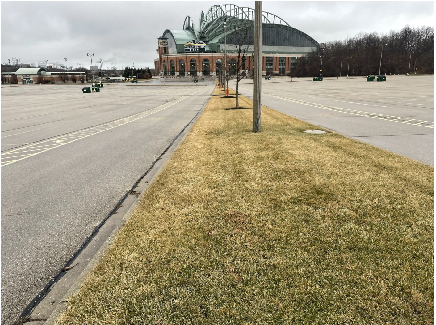
Photo 68: Money Lot: Asphalt cap Money Lot (left), asphalt cap Fingers Lot (right), greenspace cap median (center). Photo taken facing southeast on January 18, 2023.
