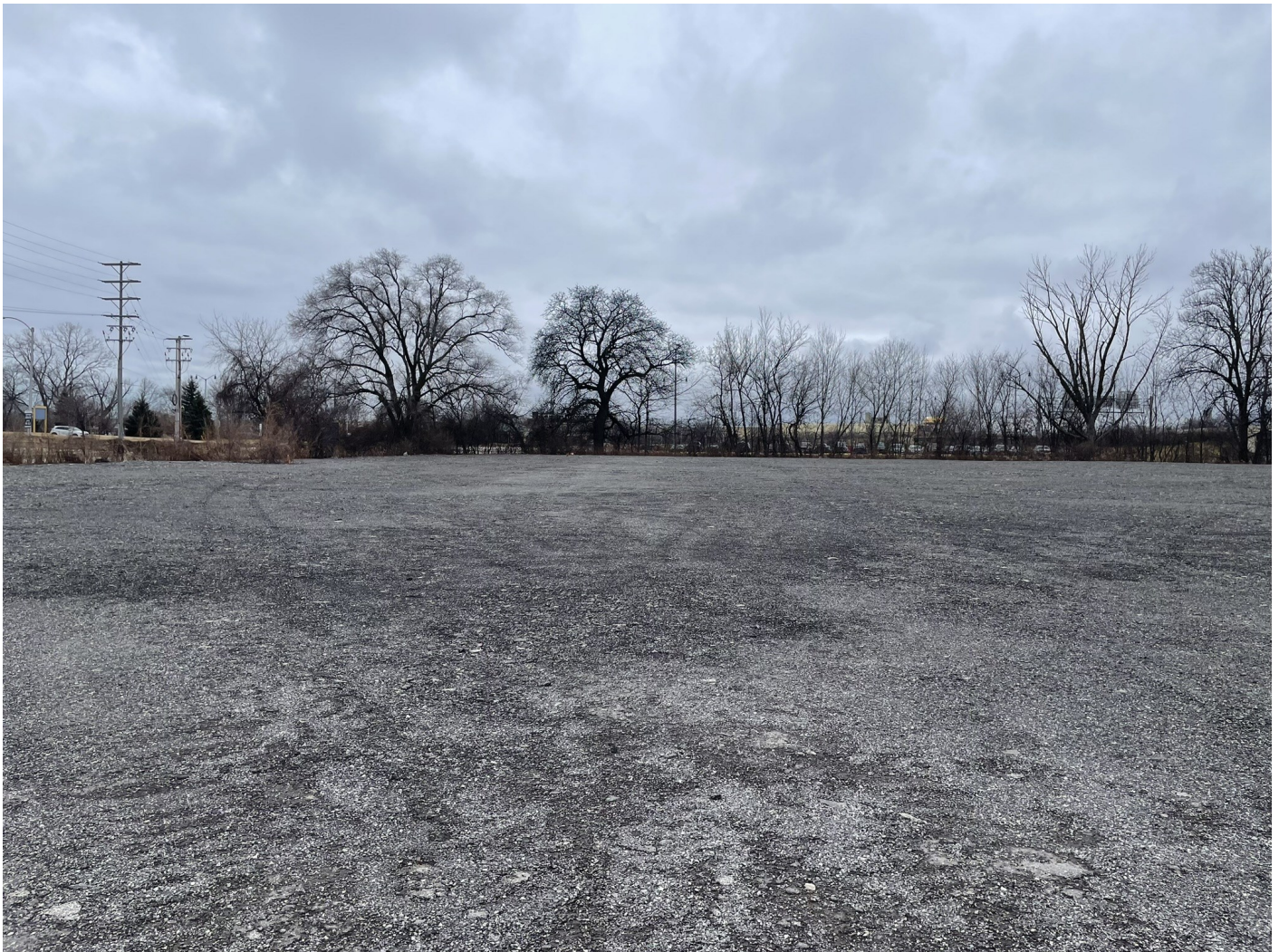
Photo 5: Staff Lot: Compacted milled asphalt cap across the Staff Lot. Between 6 and 12 inches thick. Photo taken facing south on January 18, 2023.
