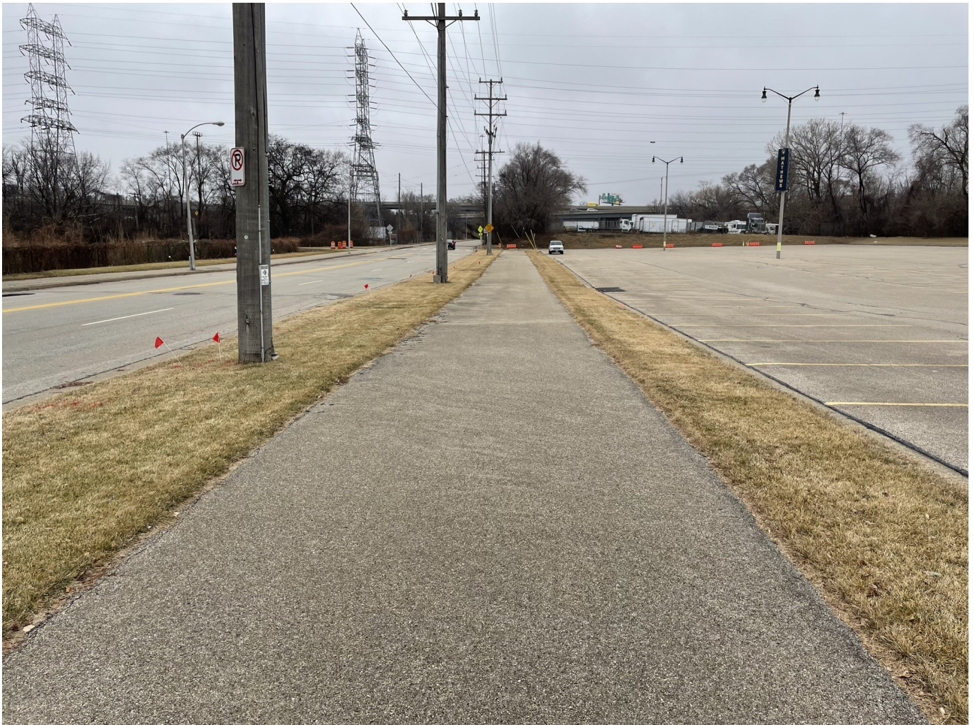
Photo 12: Matthews Lot: Asphalt cap across the pedestrian path along the western edge of Matthews Lot, representative of asphalt pedestrian path caps across the River West site. 4-inch asphalt pavement over 8-inches of crushed aggregate (base course). Photo taken facing north on January 18, 2023.
