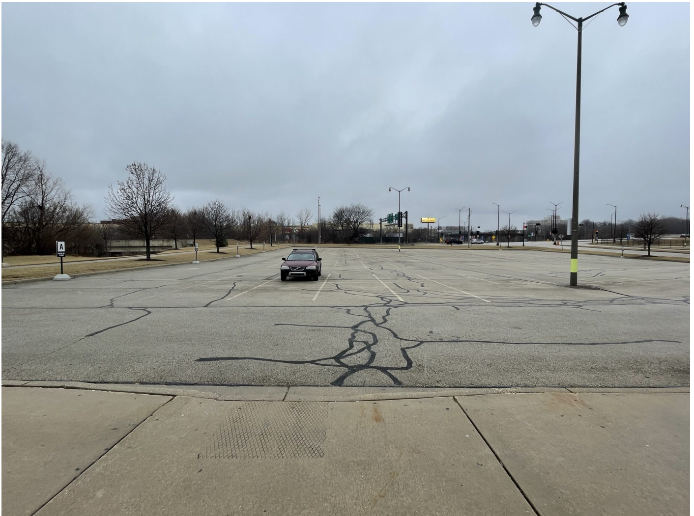
Photo 23: Ganter Lot: Asphalt cap across the entire Ganter Lot parking lot, representative of asphalt parking lot caps across the River West site. 4-inch asphalt pavement over 8-inches of crushed aggregate (base course). Concrete paved pedestrian sidewalk cap with curb and gutter cap in photo foreground. Sidewalk and curb 6-inch thick concrete, gutter 8-inch thick concrete over crushed aggregate.
