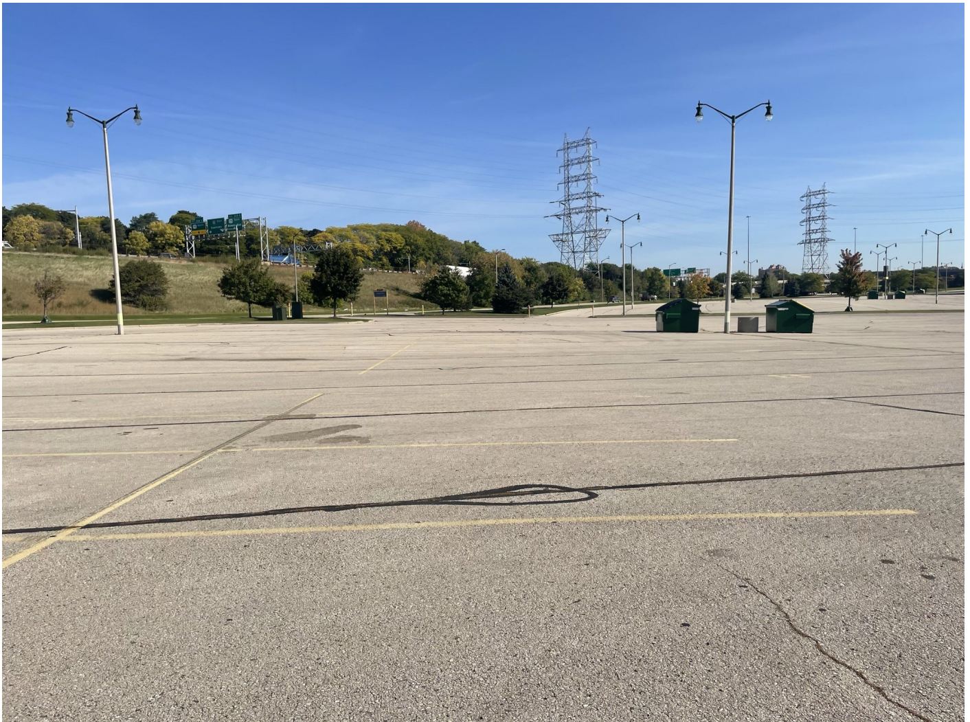
Photo 70: Fingers Lot: Asphalt cap surface lot: 4-inch asphalt pavement over 8-inches of crushed aggregate. Photo taken facing northeast on October 4, 2022.
